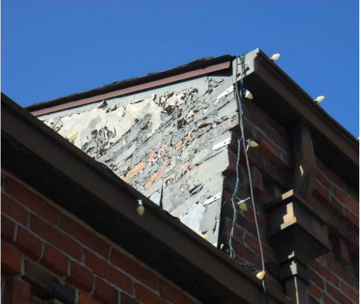
Photo 5: This is a commercial office building built in 1900 is located at 516 Main Street in Downtown Placerville. The exterior building materials are extremely damaged due to faulty weather protection and neglect. Additionally, the building has substandard exterior plumbing. According to retired City staff member Robert Shinkle, the gutters run straight into the City's sewer system, which can cause overloads to the system. A smoke test conducted by the City confirmed that the roof drains to the sanitary sewer system.
