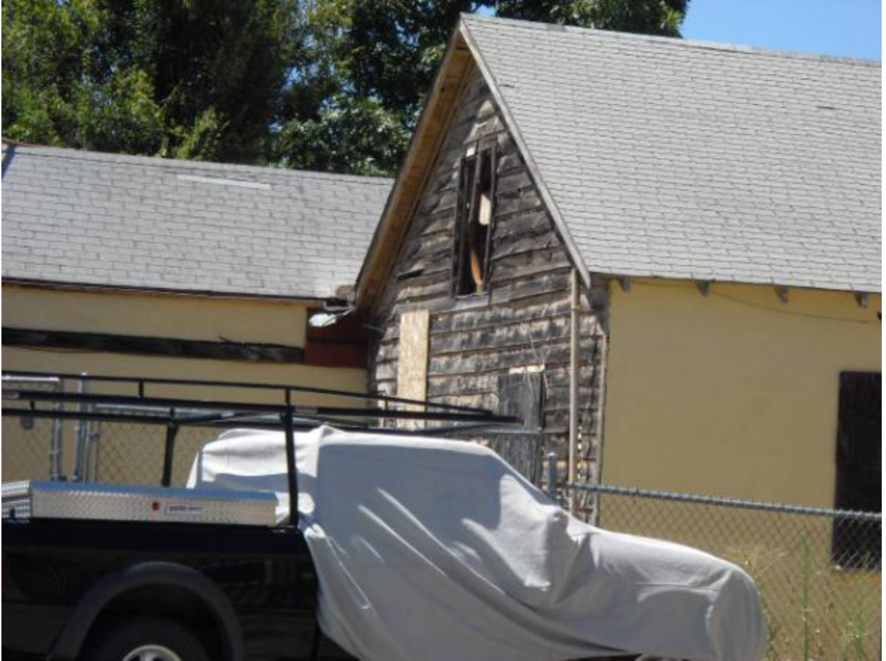
Photo 9: This commercial building at 1370 Broadway is severely dilapidated and unsafe to occupy. It has damaged exterior building materials due to faulty weather protection and long-term neglect. The wood siding at the back of the building is peeling and rotted, compromising the structural integrity of the building. Portions of the exterior wall have been patched with boards, indicating that the original wood siding provides inadequate weather protection and exposes the interior to damage from the elements.
