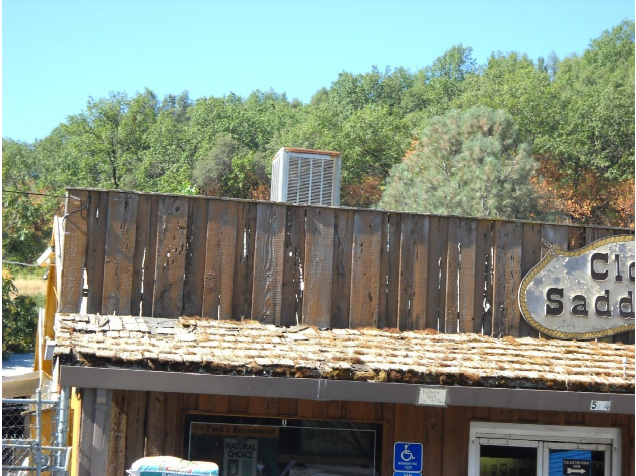
Photo 10: This building is located at 574 Placerville Drive in the Placerville Drive commercial area. A severely deteriorated roof and inadequate weather protection poses a significant threat to the health and safety of patrons and employees. According to the National Roofing Contractors Association, moss and algae growing on wood shakes causes moisture to buildup on the roof system's surface, causing accelerated rotting. Furthermore, moss and algae penetrate the roofing materials, creating cracks and crevices for water penetration.
