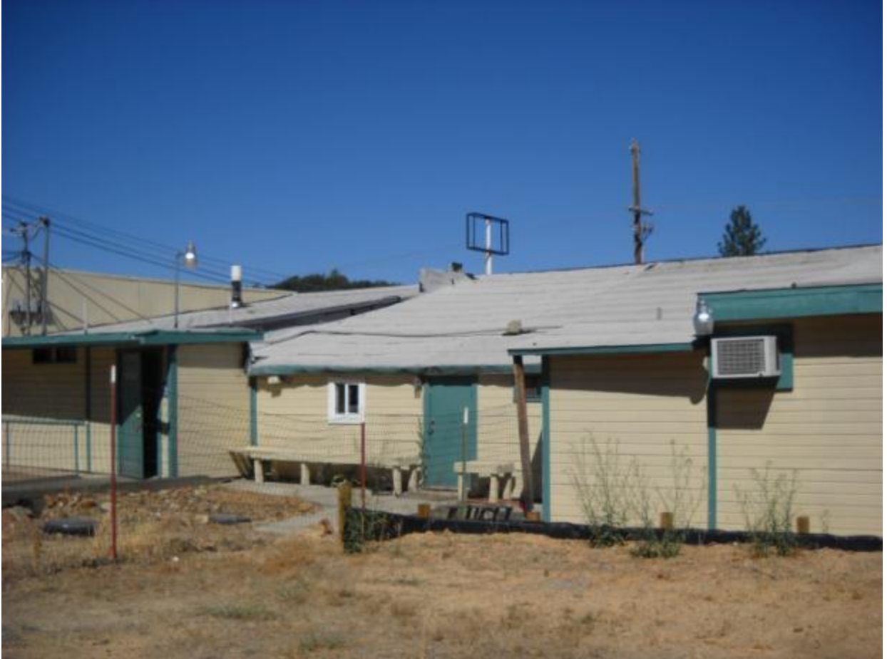
Photo 1: This commercial structure, built in 1947, is located at 418 Placerville Drive and exhibits severely damaged exterior building materials and a sagging roof. A roof in this condition indicates that the underlying structural components are compromised, weathered and dilapidated. When the structural components of a roof are flawed to this extent, the roof is a significant hazard to the health and safety of occupants.
