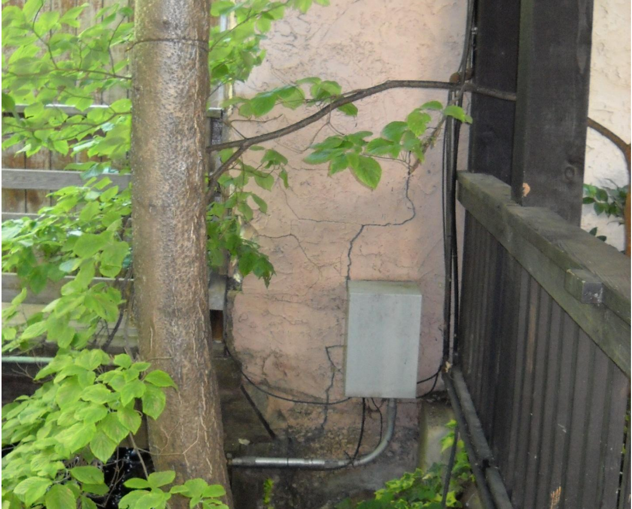
Photo 3: This building located at 459 Main Street in Downtown Placerville was built in 1886 and was vacant at the time of RSG's field survey. The cracks on the rear exterior wall indicate that the wall is falling away from the rest of the structure.
