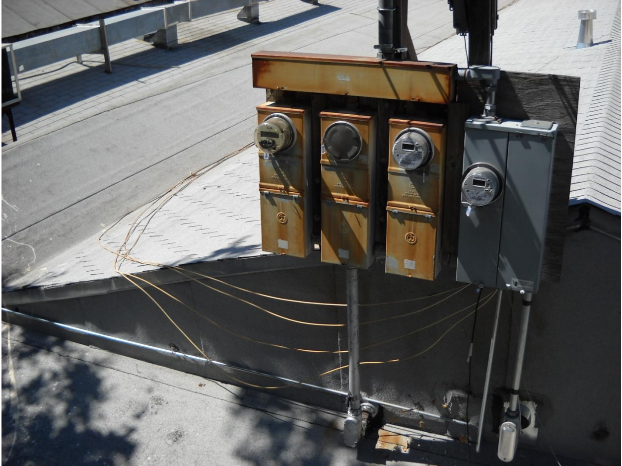
Photo 6: This is the rear of 352 Main Street in Downtown Placerville. The wiring for this structure is exposed on the roof and poses a significant health and safety hazard. The wires, extending from the electrical meter, are unsecured and running across the roof into the building. They are also within reach of the public right-of-way at Quartz Alley. Inadequate wiring poses risk of electrical shock and is a significant fire hazard.
