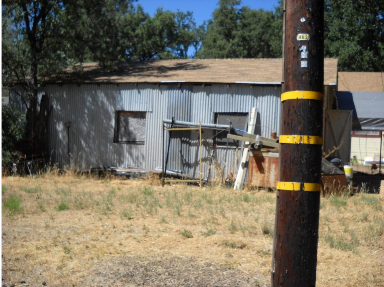
Photo 17: This structure is located on Alexander Court in the Smith Flat area of the Project Area. The building has damaged exterior building materials, as the corrugated metal siding is warped in places. The windows have been boarded with unpainted and unsealed plywood. Both conditions expose the interior to weather-induced damage, compromising the building's structural integrity.
