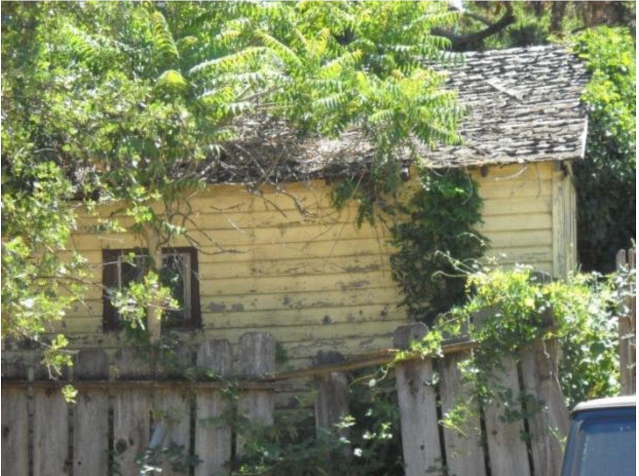
Photo 8: This building is at located at 3089 Hazard Street, near the intersections of Main Street/Spanish Ravine Road and Washington Street. This structure is severely dilapidated and unsafe to occupy. Prolonged neglect has led to broken windows, deteriorated roofing, damaged eaves and overhangs, and a significantly damaged exterior. When exterior materials are dilapidated to this extent, the interior of the structure is exposed to accelerated weathering and damage, leading to structural failure or complete collapse.
