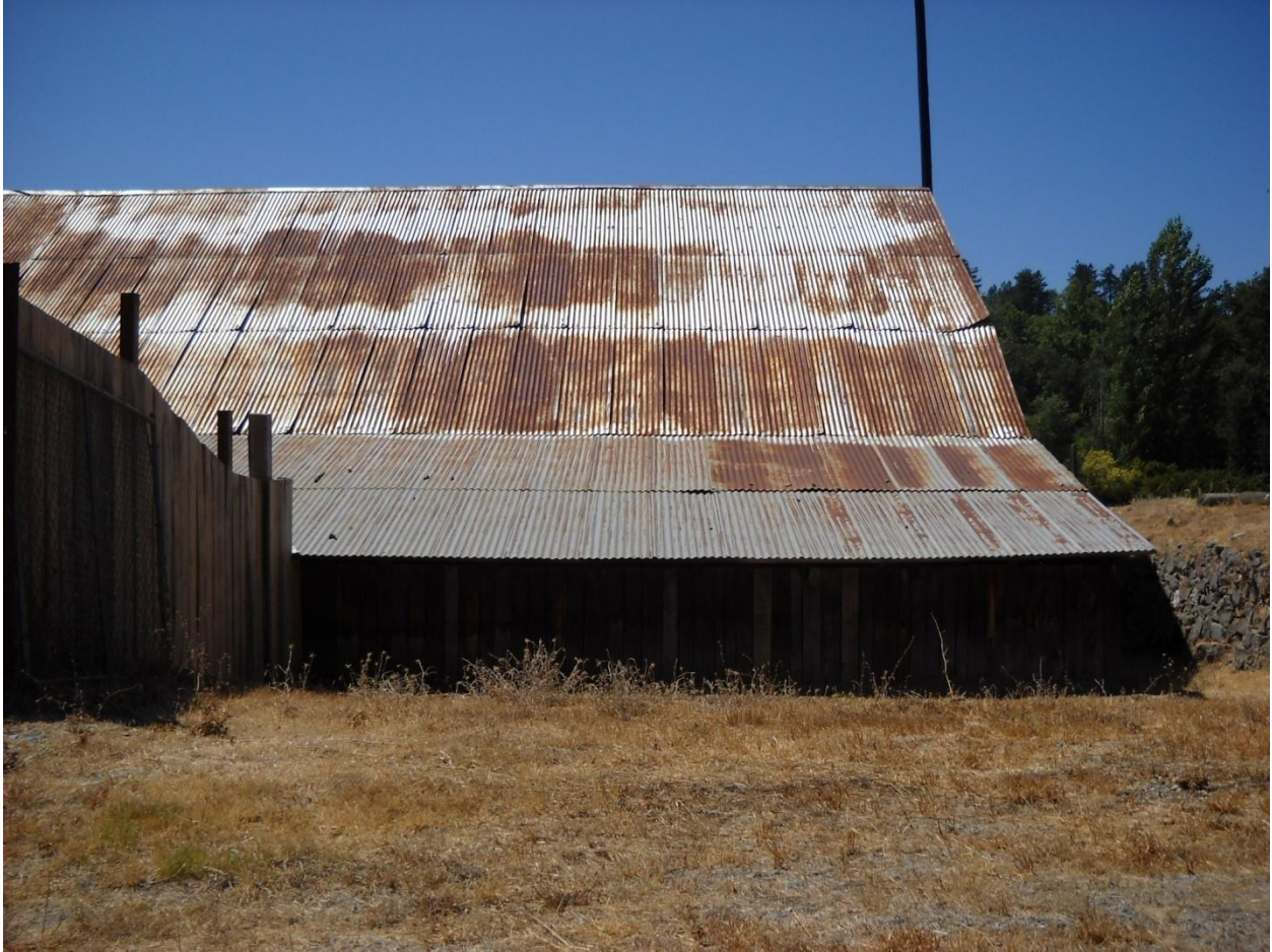
Photo 16: This building is located at 2021 Smith Flat Road in the unincorporated Smith Flat area. Portions of the walls are damaged and rotting. This roof is warped in several locations and is severely rusted, providing inadequate protection from the elements. A roof in this condition is prone to structural collapse, placing employees and patrons' health and safety at significant risk.
