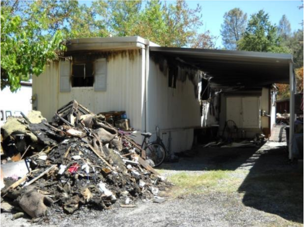
Photo 16: This residential property is located on Parkway Drive within the Motor City unincorporated portion of the Project Area. This trailer has been severely damaged in a fire and is no longer habitable. Rehabilitation is not realistic because the damage to this trailer is so extensive.
