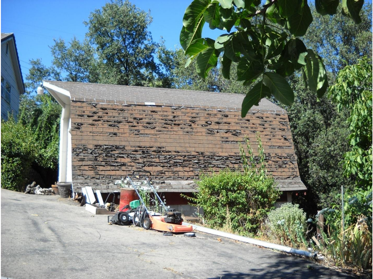
Photo 7: This building is located at 665 Placerville Drive in the Placerville Drive commercial area. It was constructed in 1940. This roof is extremely deteriorated due to long-term neglect, allowing water and moisture to penetrate the structural components of this building. Water and moisture corrode structural materials, making the building less structurally sound and leading to mold infestations. This places residents' health and safety at significant risk.
