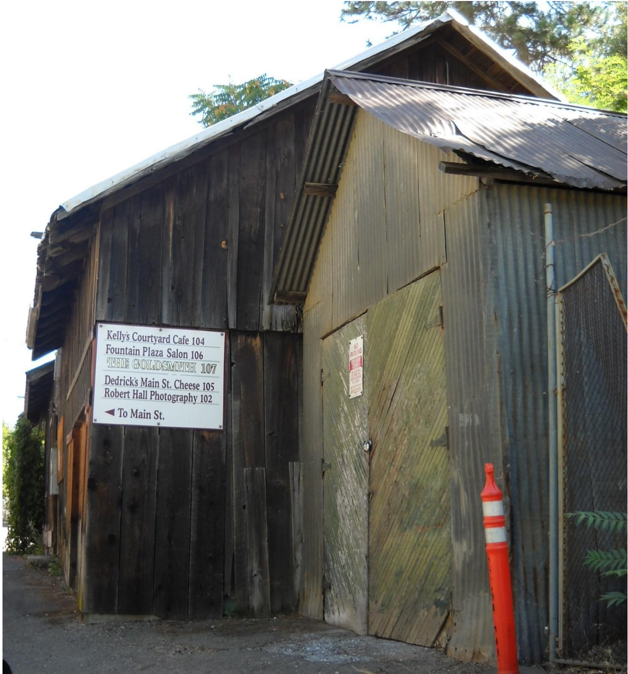
Photo 4: This building is located at 3059 Quartz Alley, south of Main Street in Downtown Placerville. Many of the buildings on this alley have been neglected for a prolonged period of time and exhibit physical conditions such as a lack of weather protection, deteriorated and damaged roofing and overhangs, and other damaged exterior building materials. This building in particular has a severely damaged roof that is warped and exposes the materials underneath to the elements. Faulty weather protection has led to a damaged exterior that is rotting and molding.
