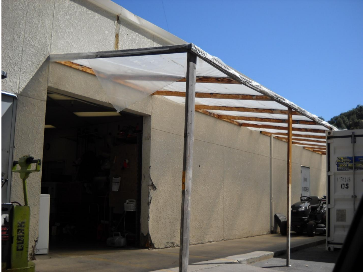
Photo 11: This is the back of a commercial store at Hillside Plaza on 384 Placerville Drive in the Placerville Drive commercial area. It has a poorly constructed overhang affixed to the building with nails with an inadequate foundation. The two-by-fours holding the overhang up are simply sitting on a parking-lot surface. The lack of an adequate foundation and poor construction is a significant health and safety concern as it can collapse on passersby.
