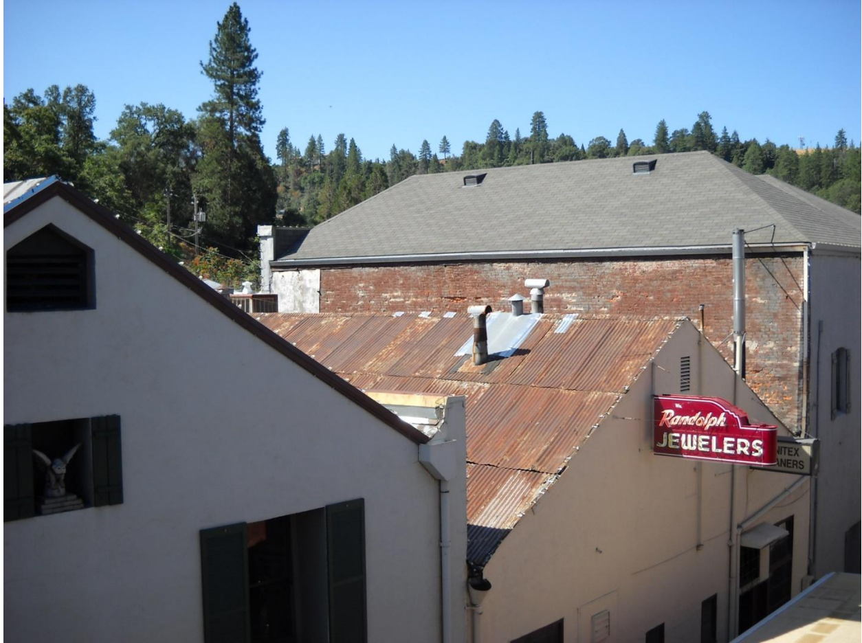
Photo 2: This is a photograph of 371 Main Street. The corrugated metal roof is deteriorated and rusted. Portions of the metal panels are warped and provide inadequate weather protection, exposing the materials underneath to damage from the elements. The bricks on the side wall are damaged and portions have fallen off the building. Falling bricks compromise the structural integrity of the building and pose a significant health and safety threat to occupants and passersby.
