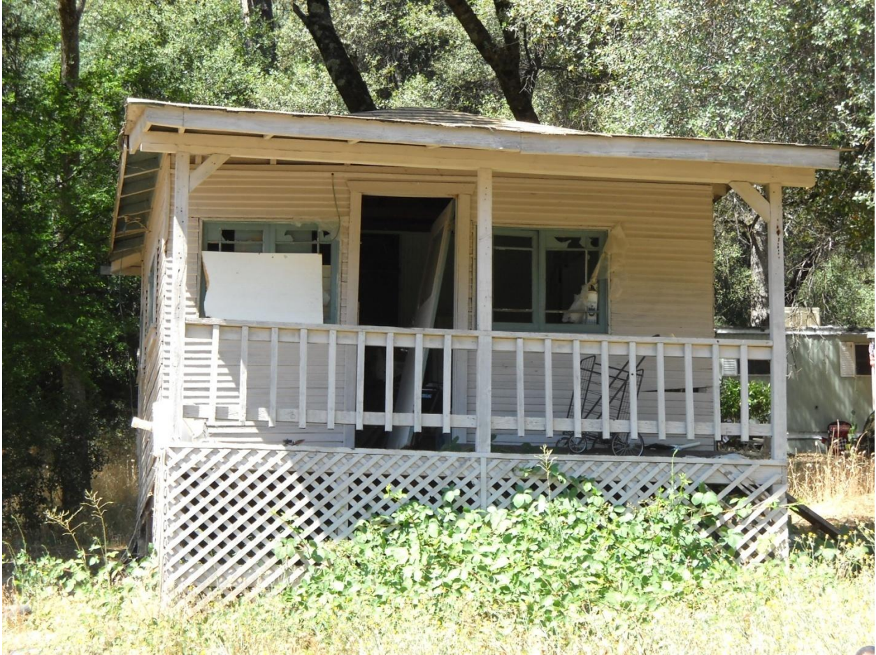
Photo 14: This structure is located on Parkway Drive in the Motor City portion of the Project Area. At the time of RSG's field survey, the building was inhabited despite having broken doors and windows, a dilapidated and sagging roof, and damaged wood siding that created holes in the exterior wall. The structure is unsafe and unhealthy to occupy because it fails to protect residents from the elements and is structurally unsound.
