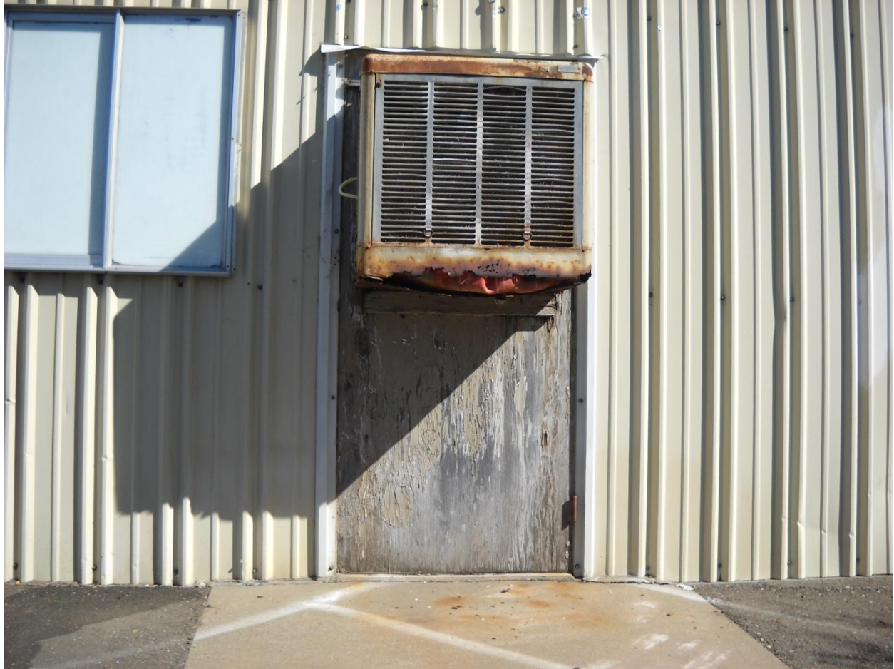
Photo 8: This commercial building is located at 175 Placerville Drive in the Placerville Drive commercial area. It was built in 1977. The building has damaged exterior building materials and exposed wiring that create a fire hazard. Substandard building materials have been used on the external shell of the building. In particular, unsealed plywood has been used in place of a door and affixed with an air conditioning unit that is severely deteriorated.
