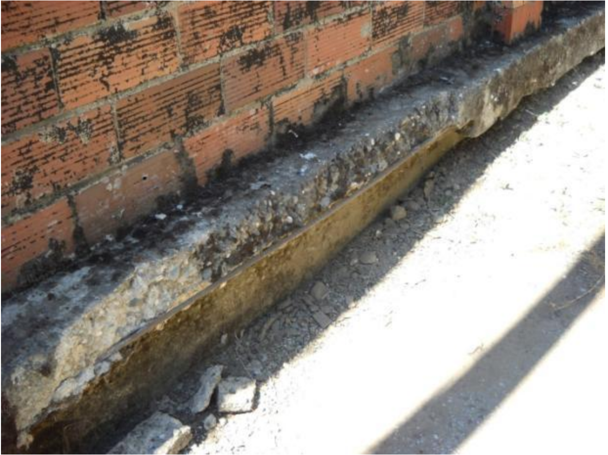
Photo 6: This is the base of a commercial structure located at 460 Main Street in Downtown Placerville. Built in 1973, the foundation of this structure has been severely damaged, leaving a pipe exposed to the elements. A damaged foundation can lead to overall structural failure and collapse.
