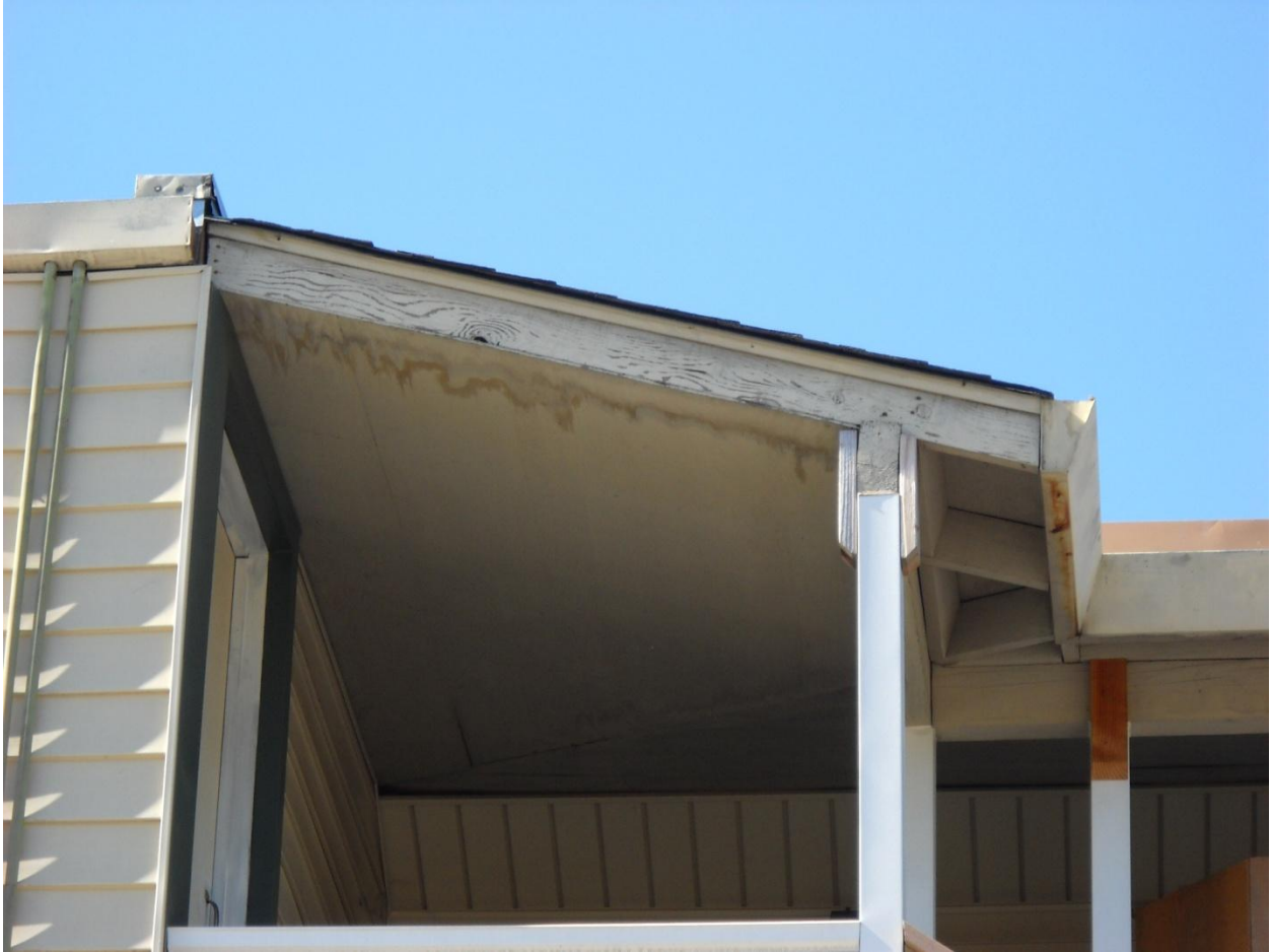
Photo 9: This building is located at 615 Placerville Drive in the Placerville Drive commercial area, near the western end of the City. This building has faulty weather protection, which has resulted in deteriorated eaves and overhangs. The picture shows the water damage that has resulted from the lack of adequate weather protection and poorly configured eaves and overhangs. Several structural supports appear to have been replaced due to water damage and the remaining structure poses a health and safety hazard to residents, patrons and employees.
