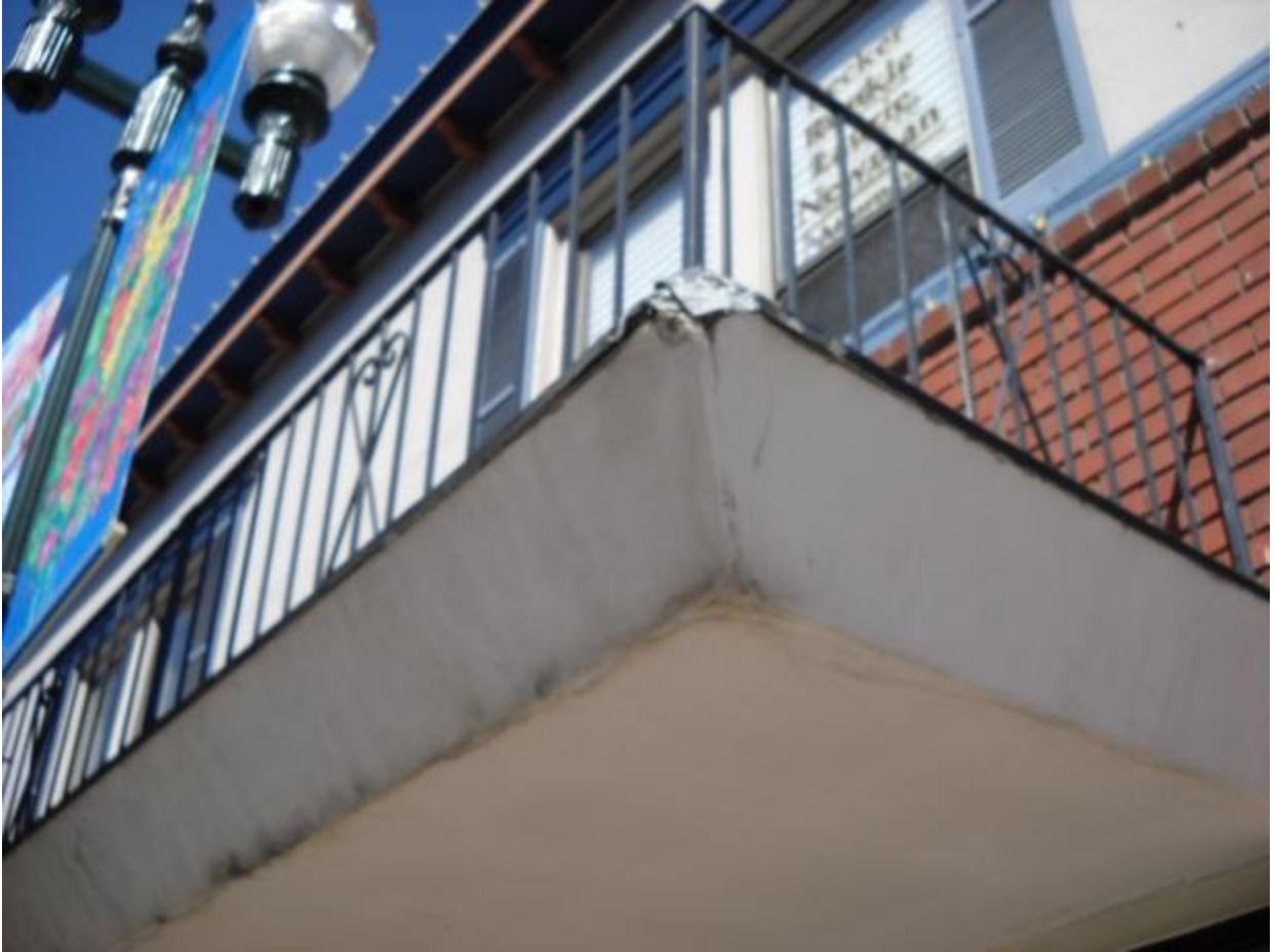
Photo 18: This is a photograph of 263 Main Street. This building exhibits signs of damaged exterior building materials and, according to retired City staff member Robert Shinkle, experiences significant flooding and dampness in the basement. Mr. Shinkle indicated that the building is currently vacant due in part to these issues. This building requires continuous pumping of the basement to alleviate flooding and dampness. These conditions are present in several buildings along Main Street in the Downtown corridor.
