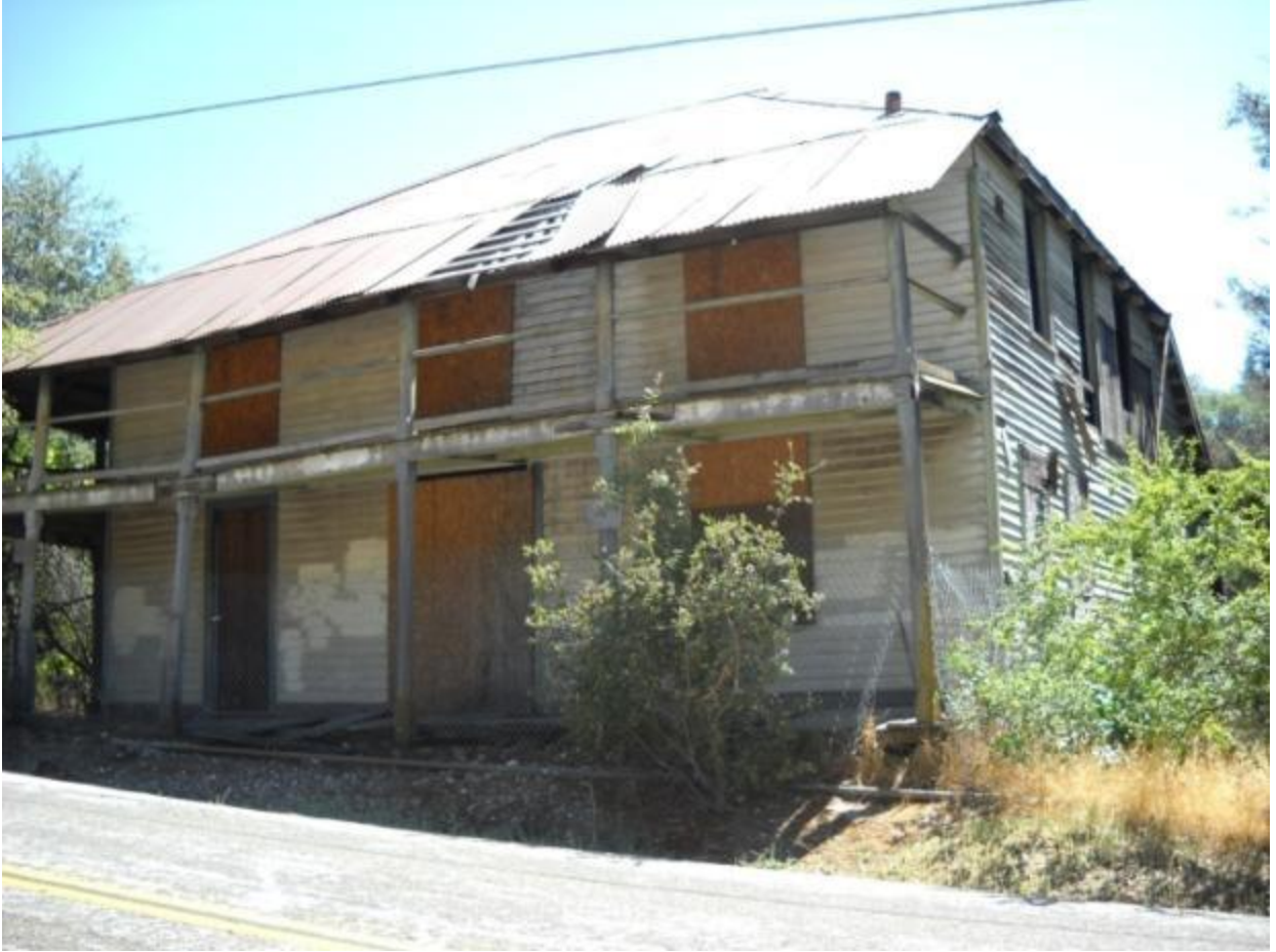
Photo 15: This structure, located on Smith Flat Road in the unincorporated Smith Flat area of the Project Area, was built in 1897 and exhibits extensive physical damage. The roof, eaves and overhangs, and other exterior building materials are broken and deteriorated. Lack of adequate weather protection exposes the interior building materials to damage and compromises the structural integrity of the building. Structures in this condition are unsafe to occupy due to structural failure and risk of collapse. Boarded doors and windows indicate that the building is vacant.
