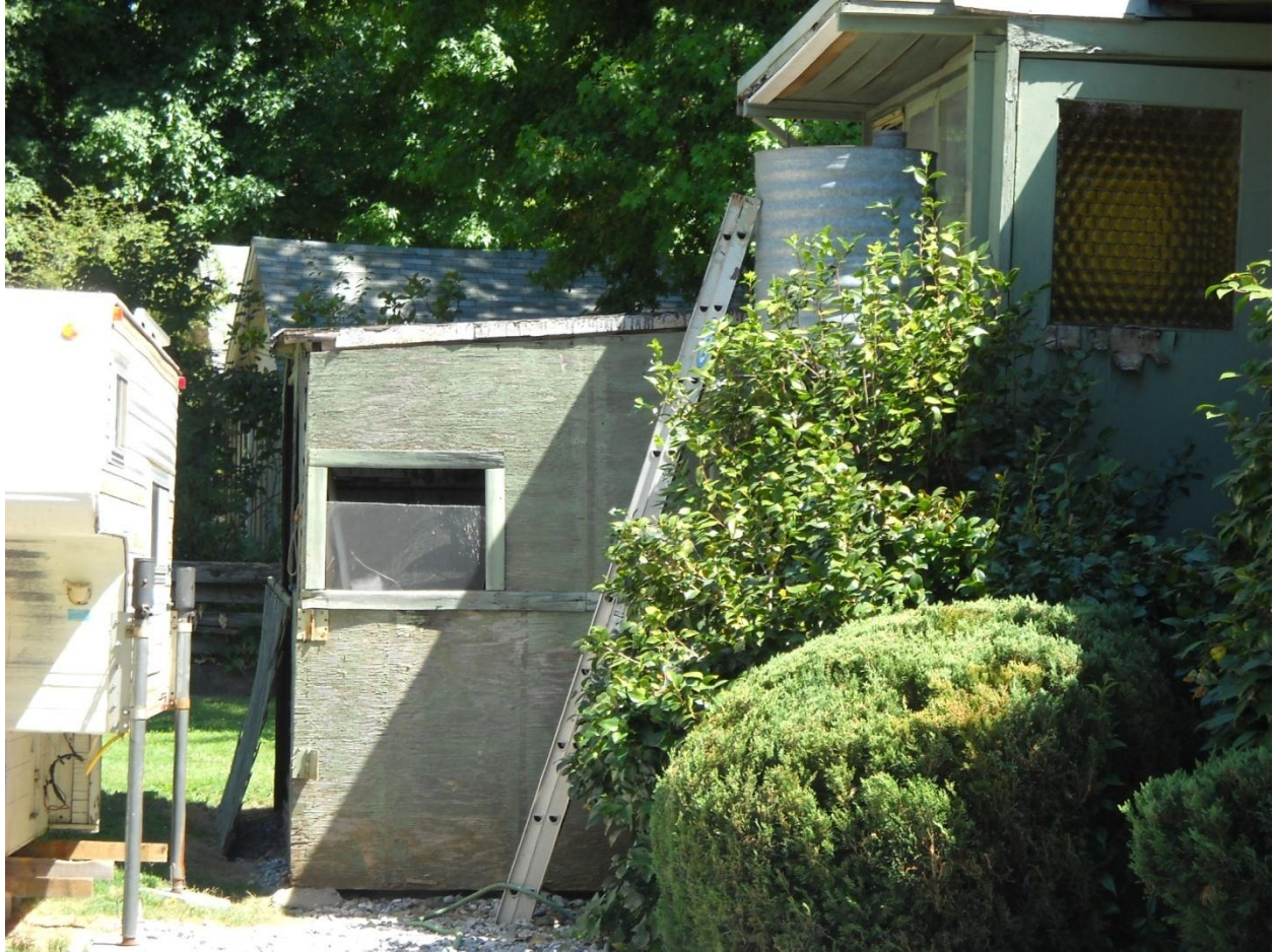
Photo 15: This building is located at 2915 Jacquier Road in the Smith Flat portion of the Project Area. The addition on the side of the property is poorly constructed with untreated plywood. The exterior building materials are damaged and have faulty weather protection, accelerating weather induced damage.
