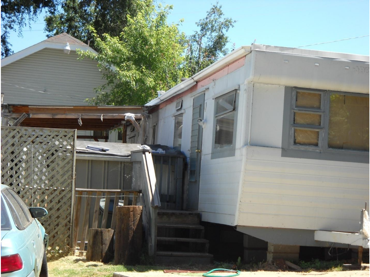
Photo 12: This mobile home is located at 3076 Washington Street near Downtown Placerville and the Broadway commercial area. The mobile home is supported by cinder blocks, which does not provide an adequate foundation. The mobile home is buckling down toward the right. The structure is not safe to occupy due to risk of collapse.
