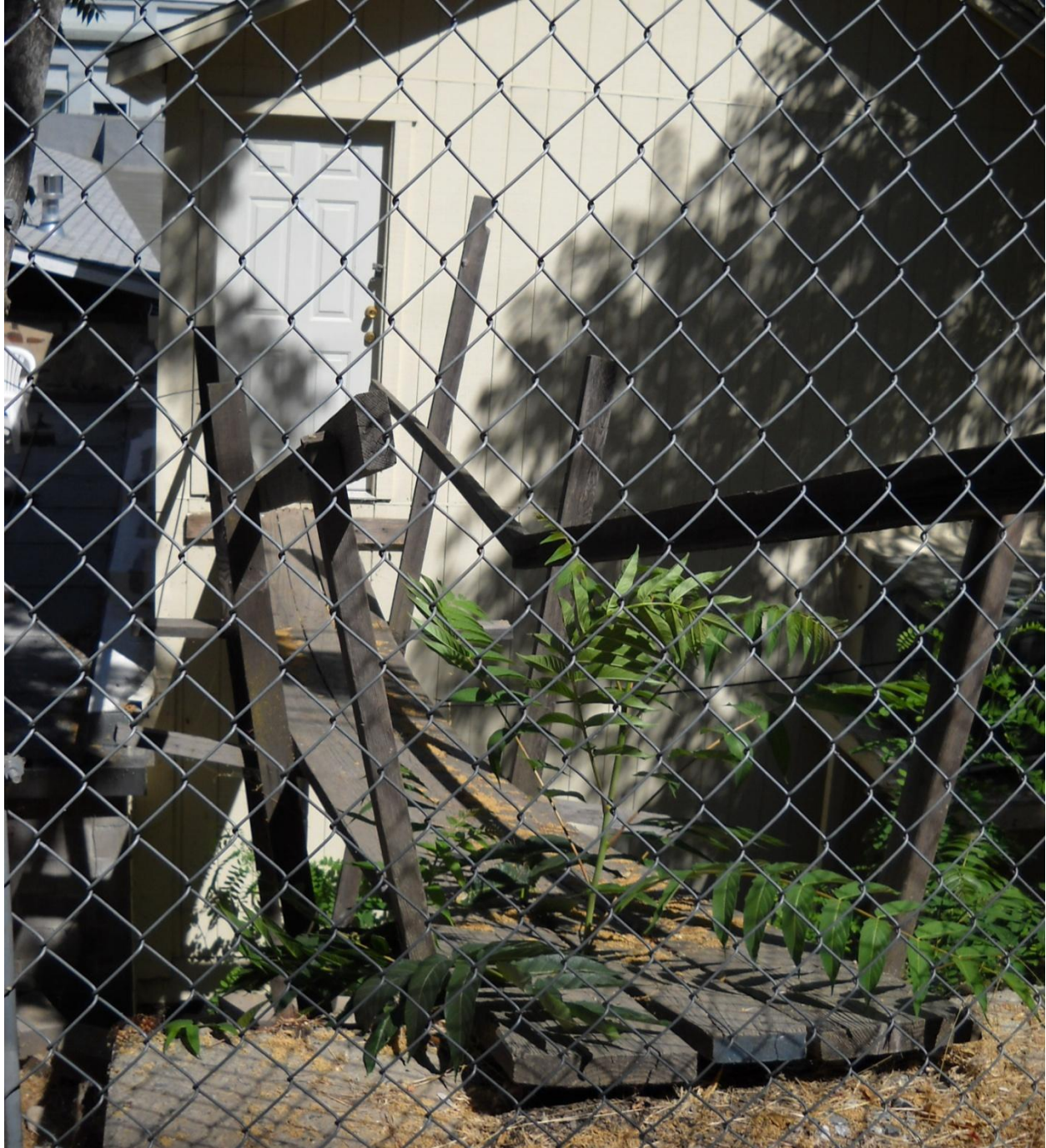
Photo 5: This footbridge is located behind 360 Main Street in Downtown Placerville. The bridge connects the second story of 360 Main Street to Quartz Alley. This bridge is poorly constructed and is a significant safety hazard, as it may collapse at any time.
