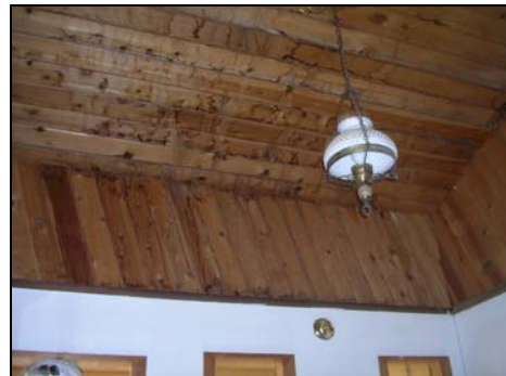
Water damage to the ceiling.
