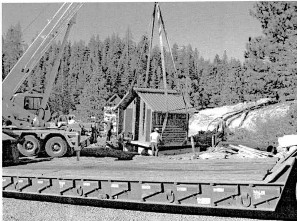
Installation of new double-vault waterless restroom at Rubicon Trail Loon Lake Trailhead
