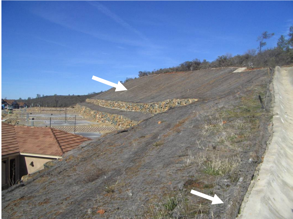
Photo 3. View of the slopes that received the Pine Hill ceanothus plantings on the east side of the Project, about a year after planting. The Pine Hill ceanothus are too small to be clearly evident in the photo. Parts of the irrigation system can be seen (arrows; 15 January 2009).
