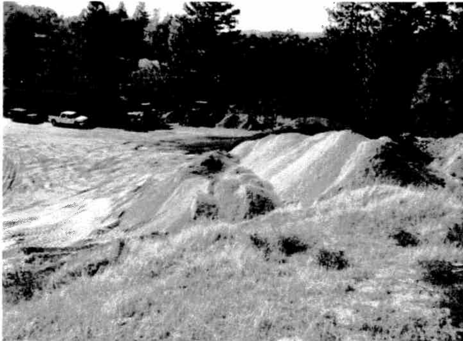
Photograph No. 1. Overburden stockpile (foreground), processed sand stockpile, equipment maintenance and storage building, imported aggregate and recyclable asphaltic material stockpiles, equipment staging area and truck loading area (viewing west).
