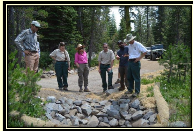
One of the newly constructed catchment basins on the lower section of 14N39, Richardson Road. Public tour of project.
