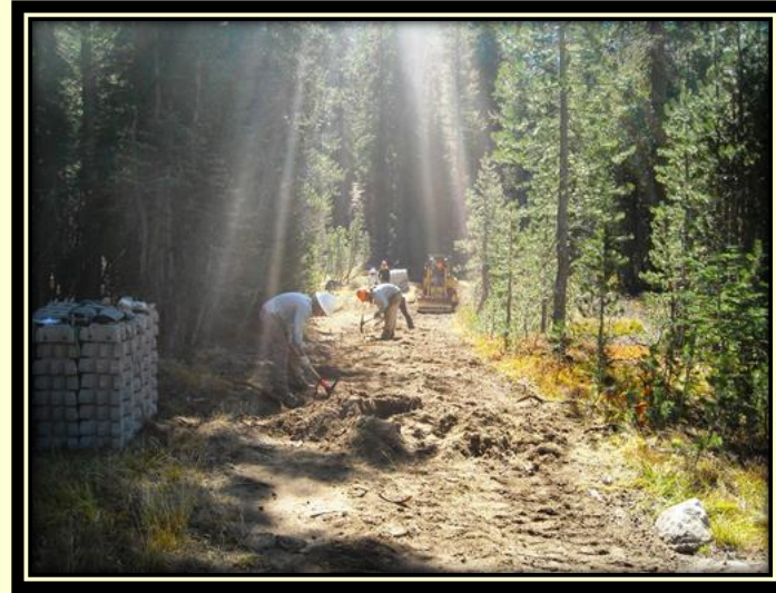
SCA Crew 5 at work in the early morning preparing grade for the block work at Meadow 6
