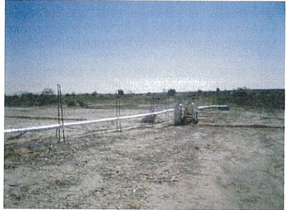
FIGURE 6 BOILER FOR EW-2 AND EW-5
