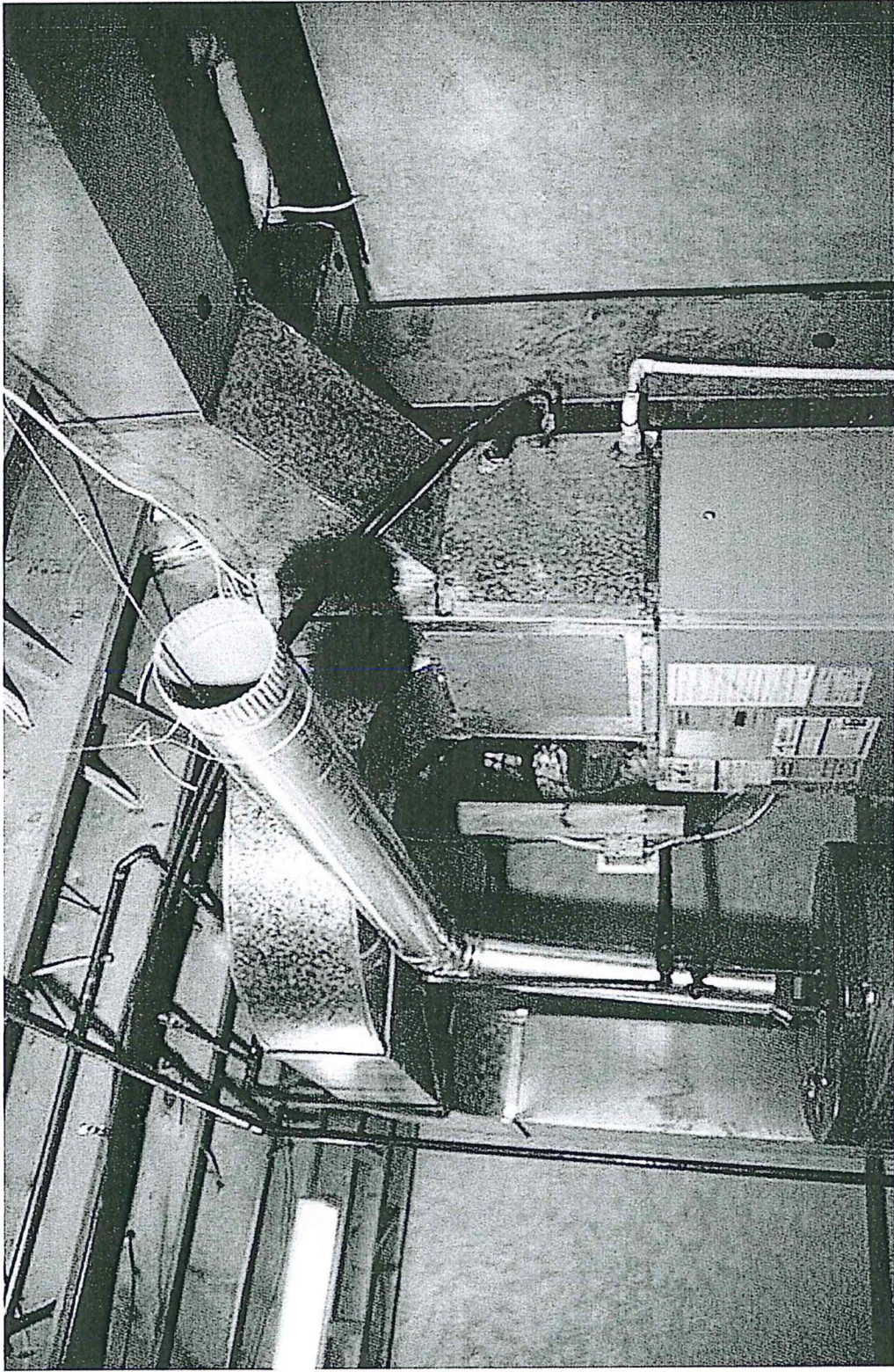
Gas Water Heater Vented into Room instead of Outside (for more CO2)
