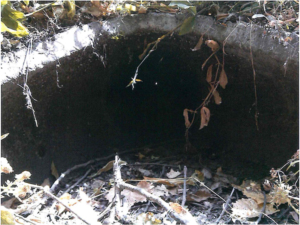
Open to down slope to concrete ditch.
