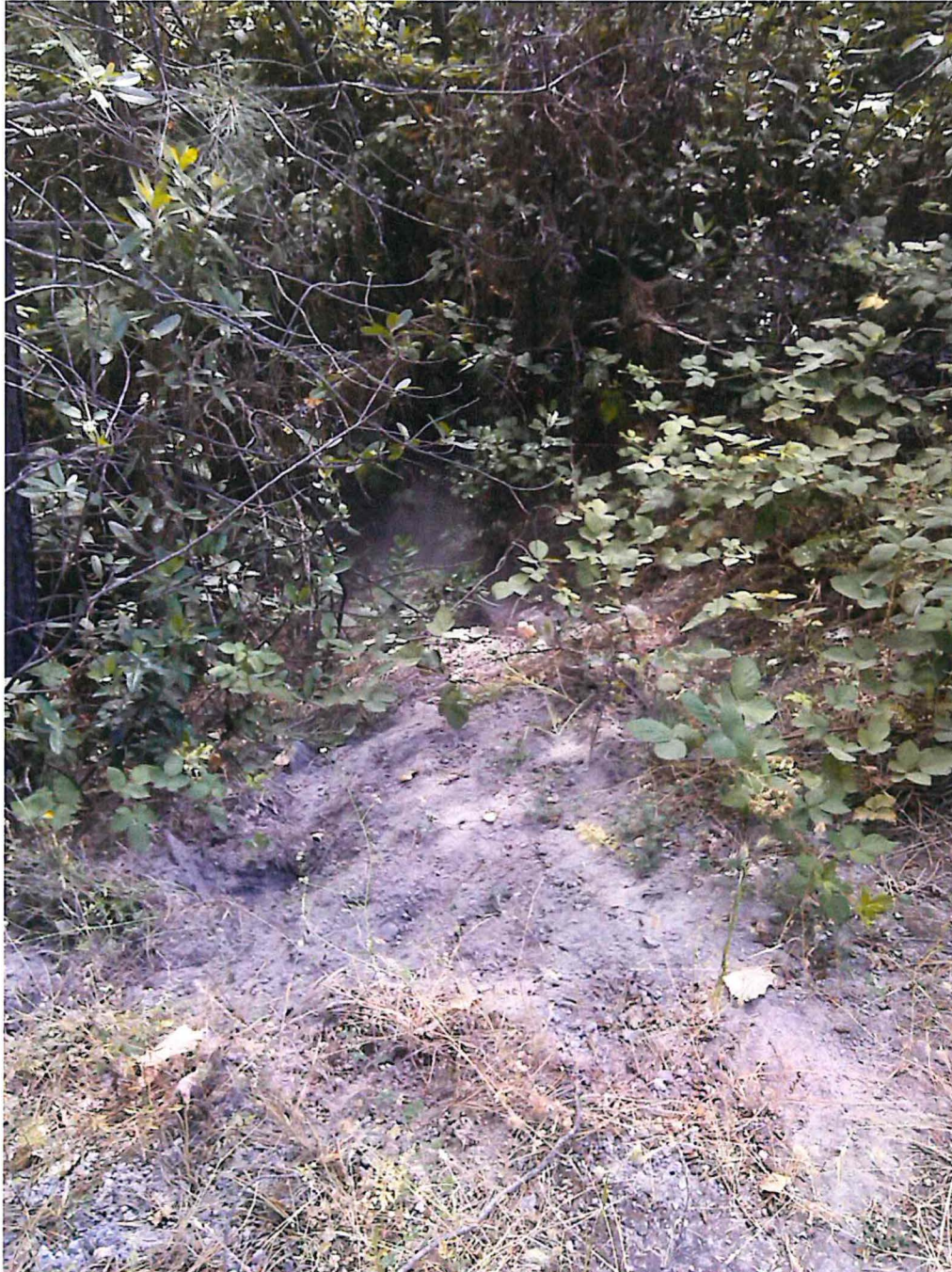
Notice toe to creek where lime slurry dumps into it from Waste Connections polluted property.
