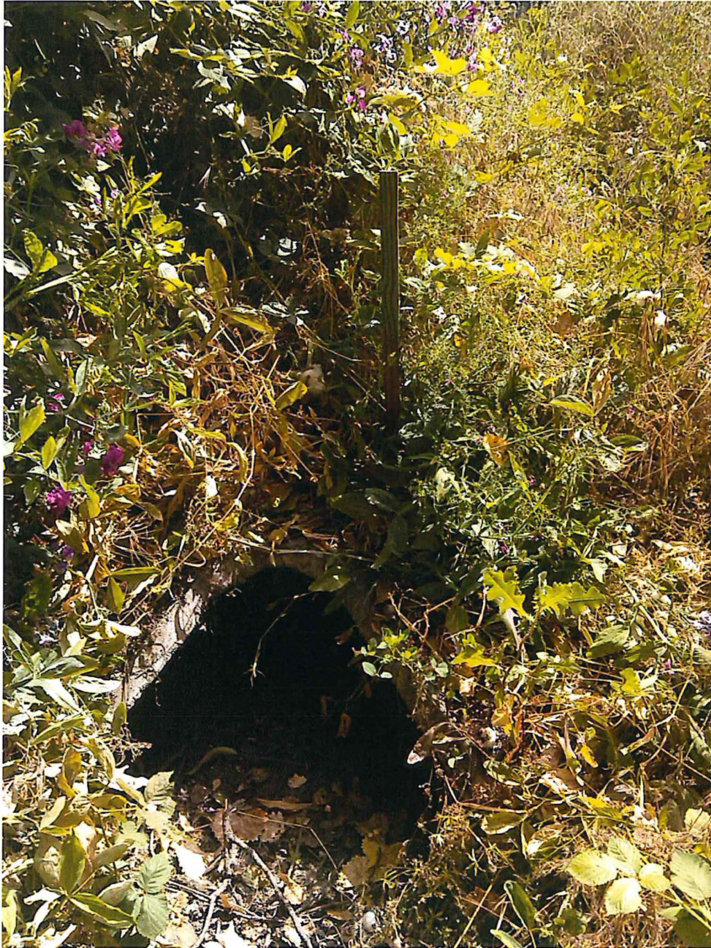
Drain inlet from Pond #2 to pond #1 shown as dashed line on faulty SWAPPP
