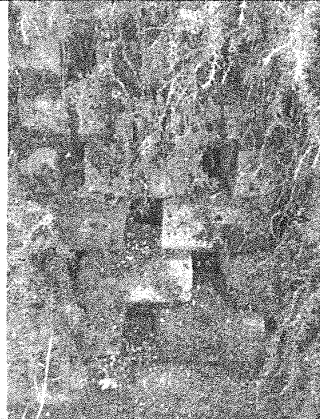
Photo 3. Detail of block wall shown in Photo 2. Rosemary plants cascading down face of wall. 20 July 2020
