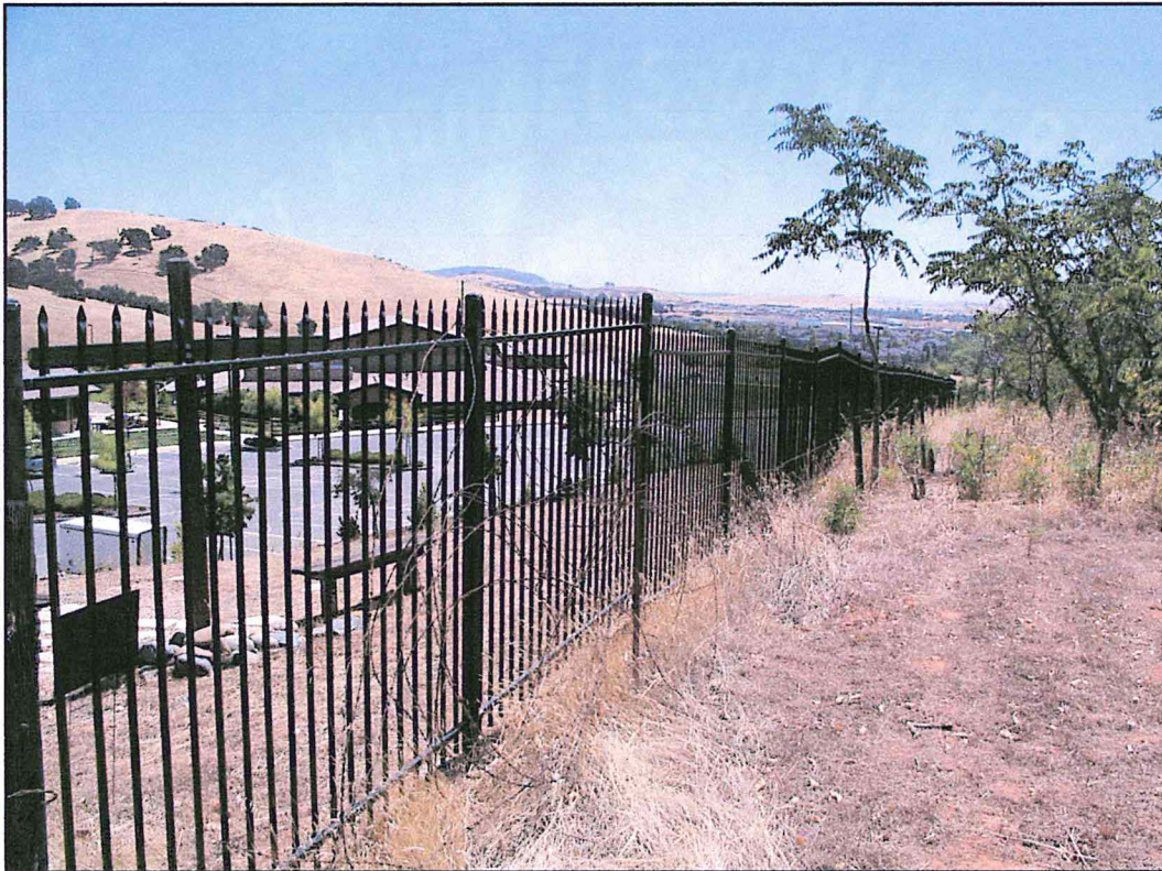
Existing wrought iron fencing installed by Lakehills Covenant Church, the style of which will be duplicated with the new fencing.
