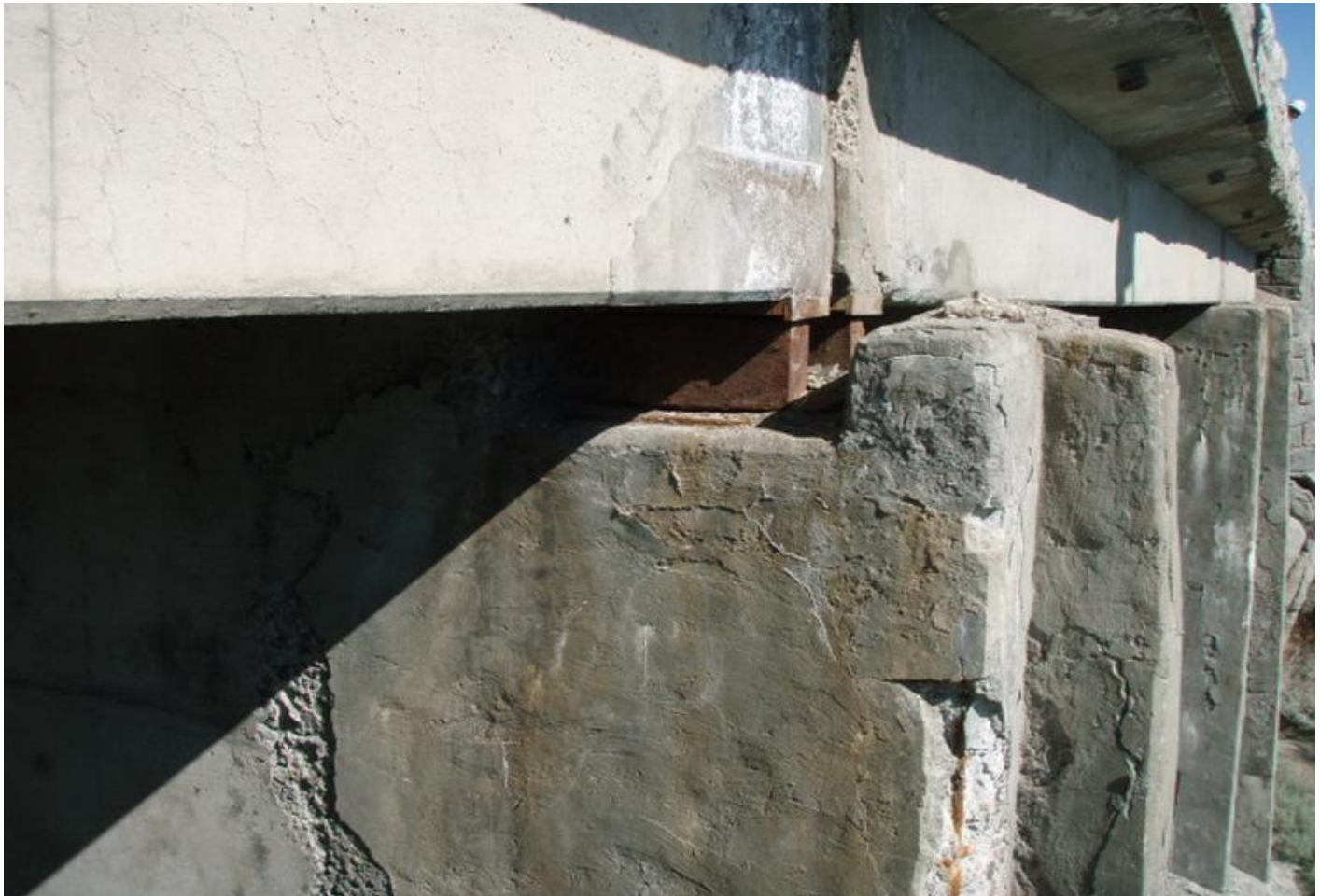
Concrete spalling in pier walls
