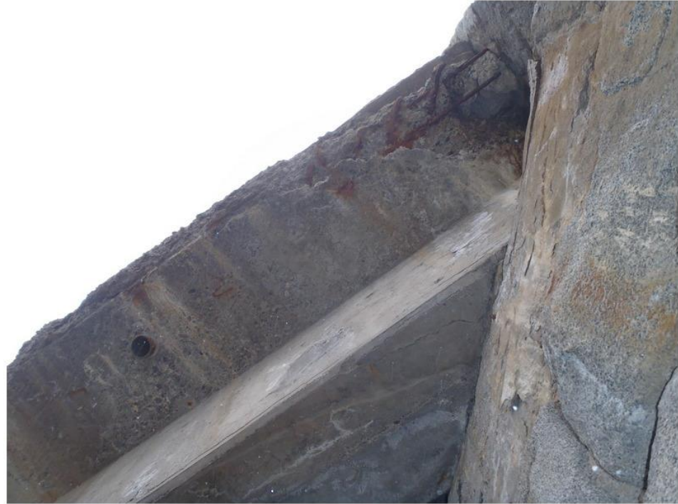
Concrete cracking and exposed reinforcing steel in girders and deck
