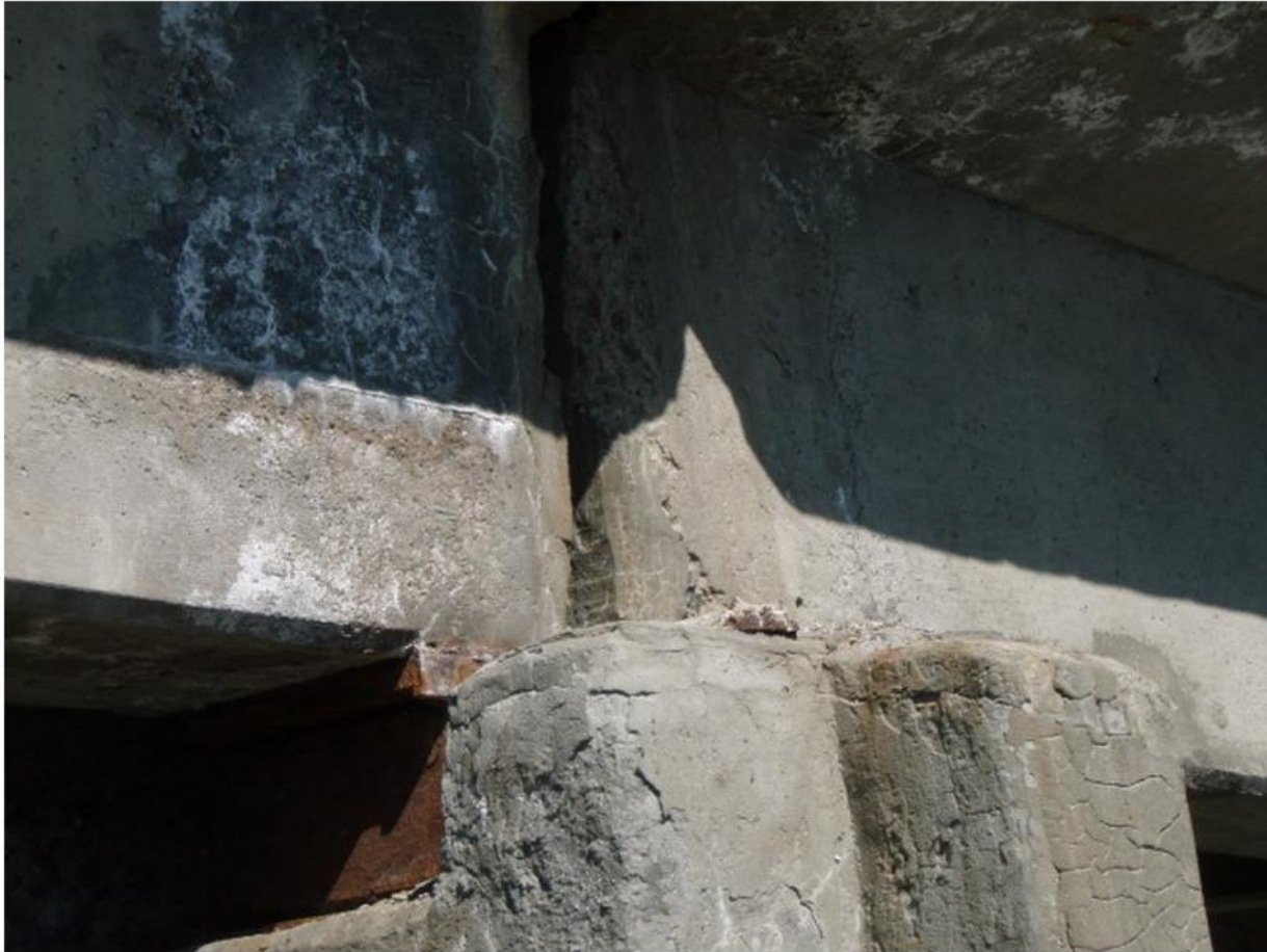
Concrete cracking and spalling in girders and piers
