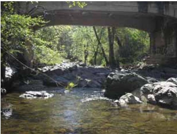
Photo 5. View looking east from the west side of Green Valley Road Bridge. 17 April 2008
