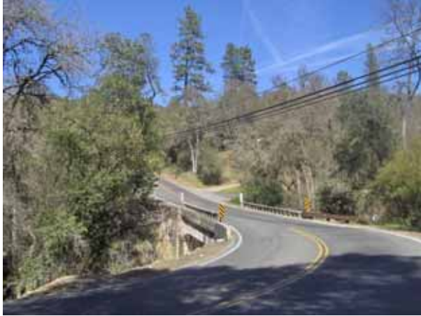
Photo 1. View looking north along the Green Valley Road Bridge (25C-0088) at Weber Creek. 27 March 2008.
