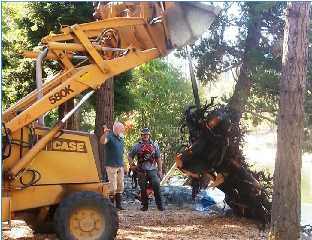
Photo 3. Tree hazard above Hwy 49 Bridge removed by backhoe
