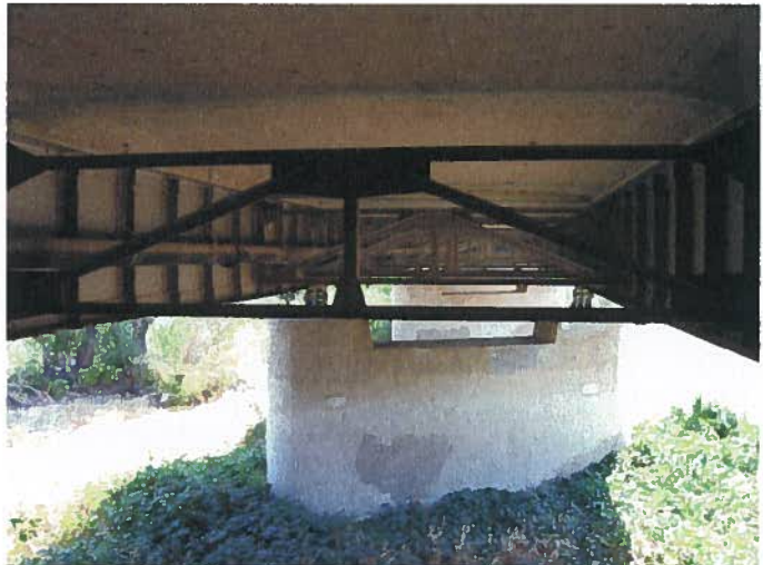
Underside of bridge deck, showing existing bracing of steel beams and connections to concrete piers.
