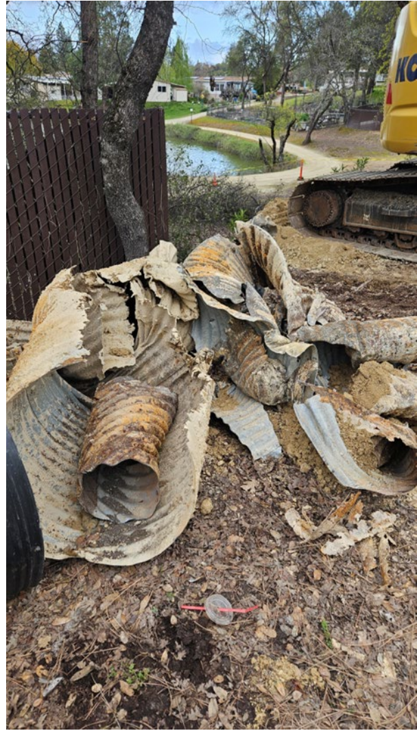
Damaged/destroyed culvert removed from roadway
