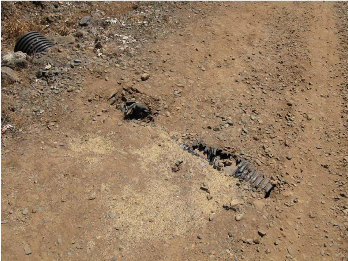
One of the drainage pipes needing repair/replacement along the Project site.
