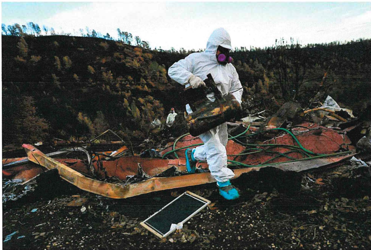
An EPA contractor carries metal material out of a property that was destroyed in the Camp Fire in Paradise, California, on Wednesday, December 5, 2018. (Photo by Gabrielle Lurie / The Chronicle)
