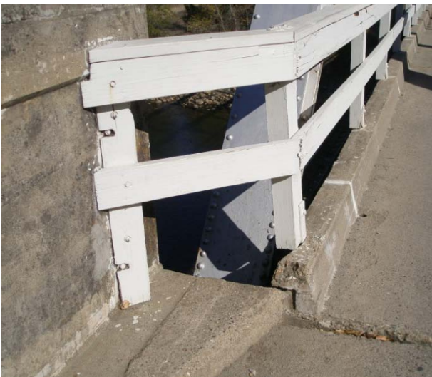
Figure 3 - Expansion joint at end of truss spans showing sub-standard approach, barriers and transition
