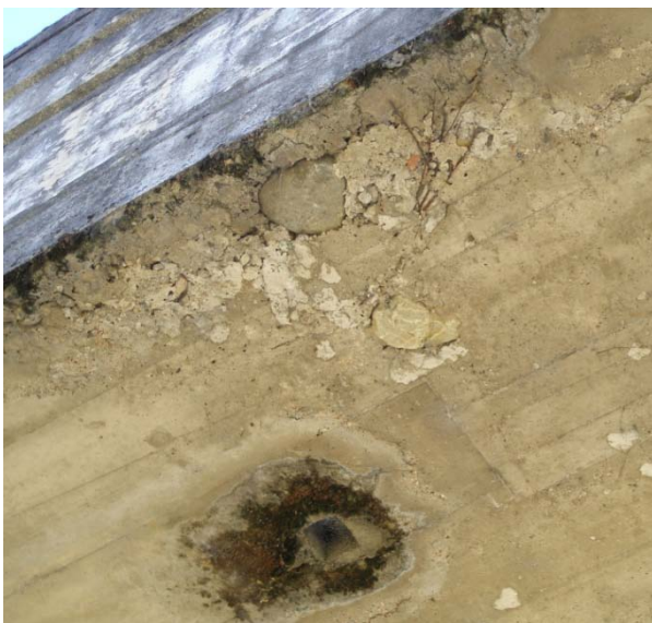
Figure 4 - Exposed large aggregates on underside of approach spans
