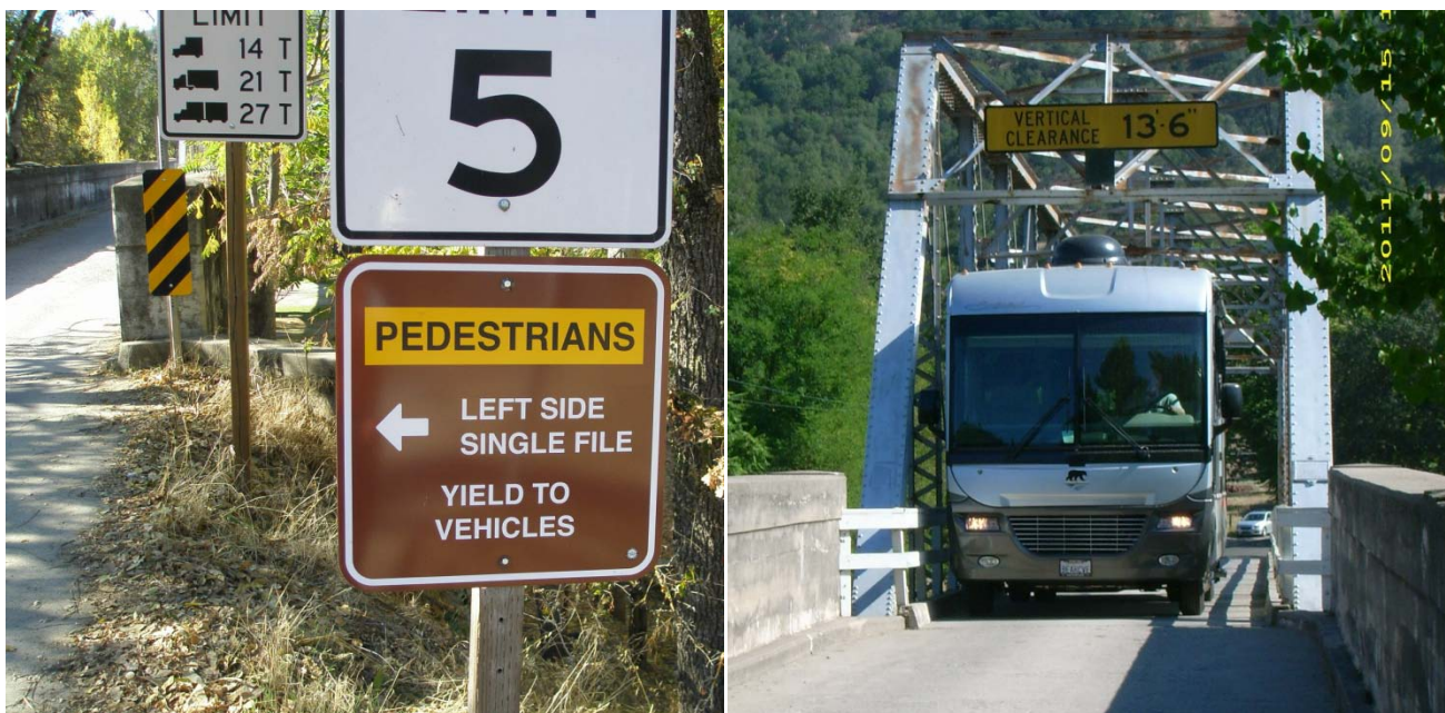
Figure 1 - Structurally Deficient and Functionally obsolete: shared vehicular and pedestrian use and posted truck loads
