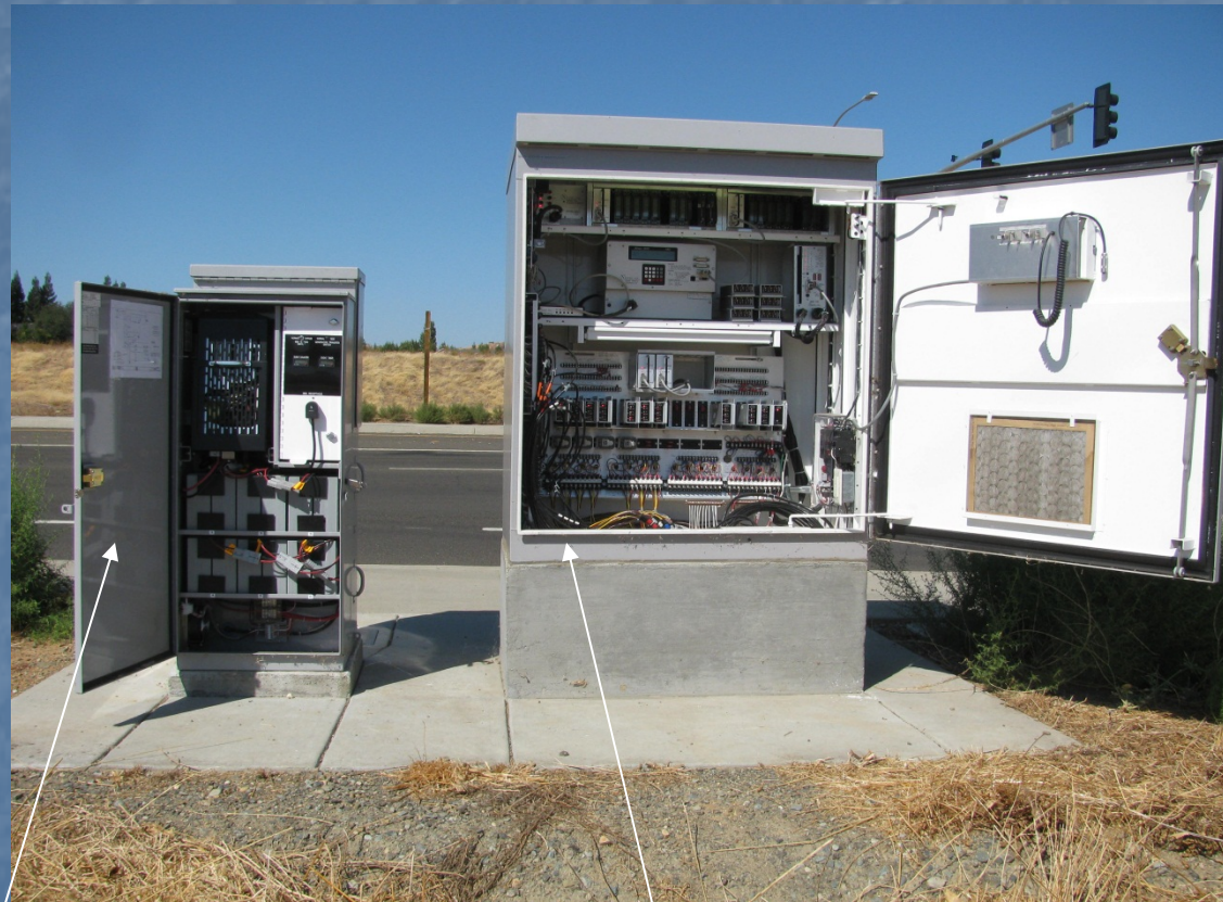
Signal Power Service and Battery Back-up Assembly
