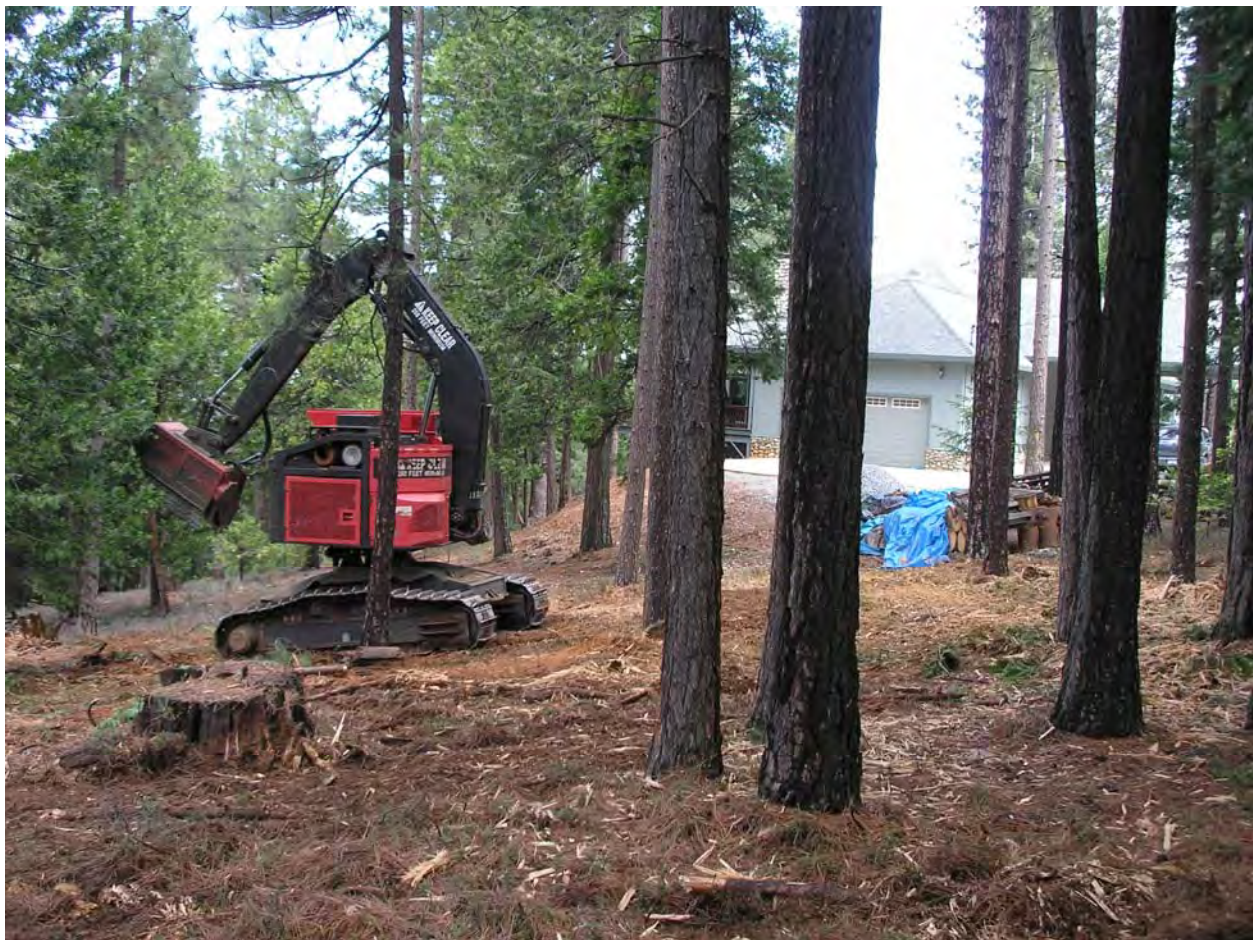
Photo 1. A rotary masticator chipping small trees and shrubs on the Grizzly Flat Fuel Reduction Project
