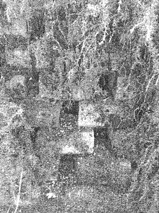
Photo 3. Detail of block wall shown in Photo 2. Rosemary plants cascading down face of wall. 20 July 2020
