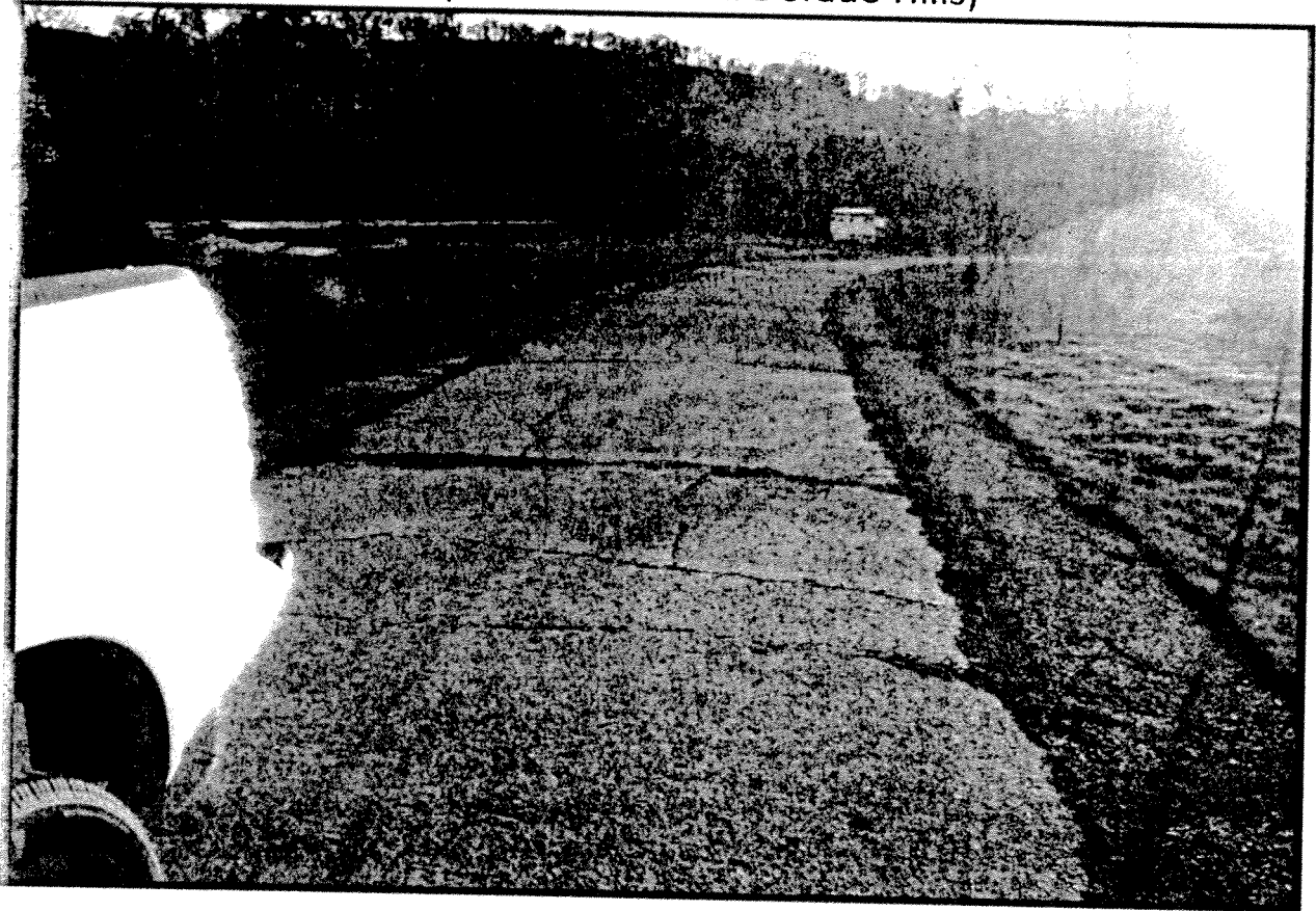
Old Lincoln Highway Cracking Example (This photo taken in El Dorado Hills)
