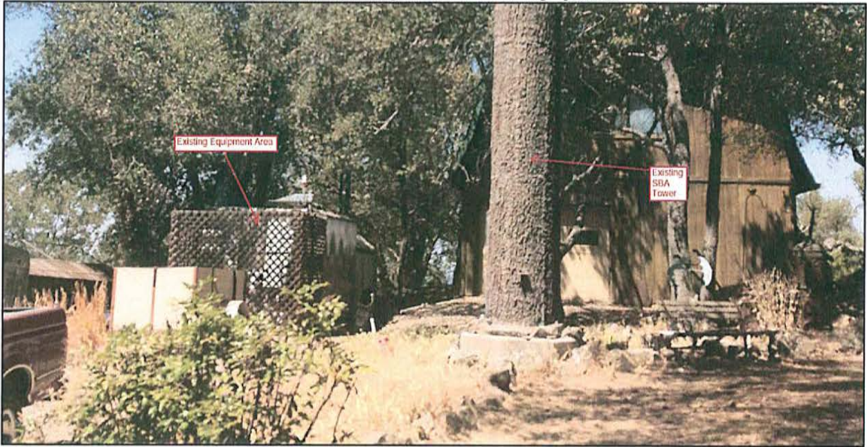
Photo of Existing SBA Ground Equipment
