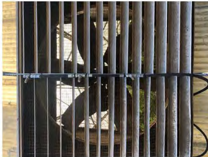
Figure 10 Details of Odor Control Misting Nozzles
