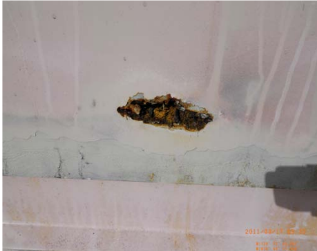
Photo 7. Rust hole on the side of container.
