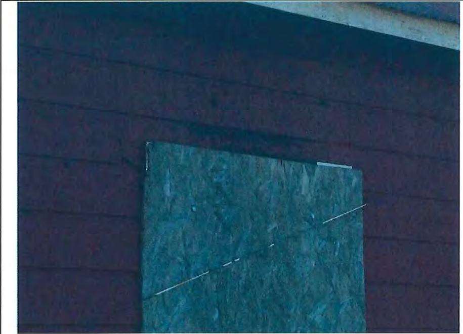
4. View looking west at the east elevation upper wall of the school, with a bee hive that has penetrated the inner wall above the boarded-up window.
