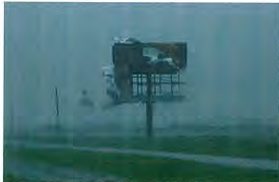
Wind and rain from Hurricane Lili damage road signs along I-10 in Louisiana on October 3, 2002
