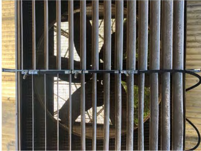
Figure 10 Details of Odor Control Misting Nozzles
