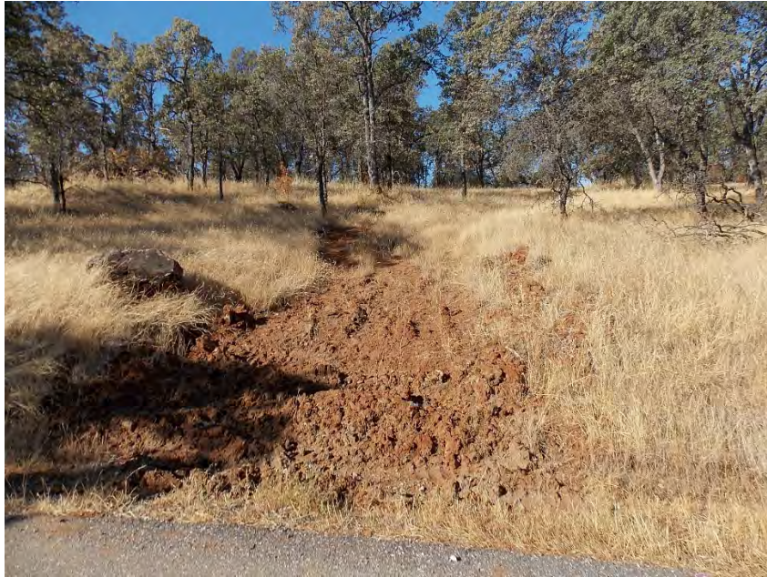
Photo 1. View from the east end of the BSA up the hill towards the southwest. This photo shows the disturbed area and the site of the future gravel access road. 13 July 2017.
