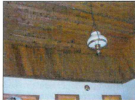
Water damage to the ceiling.
