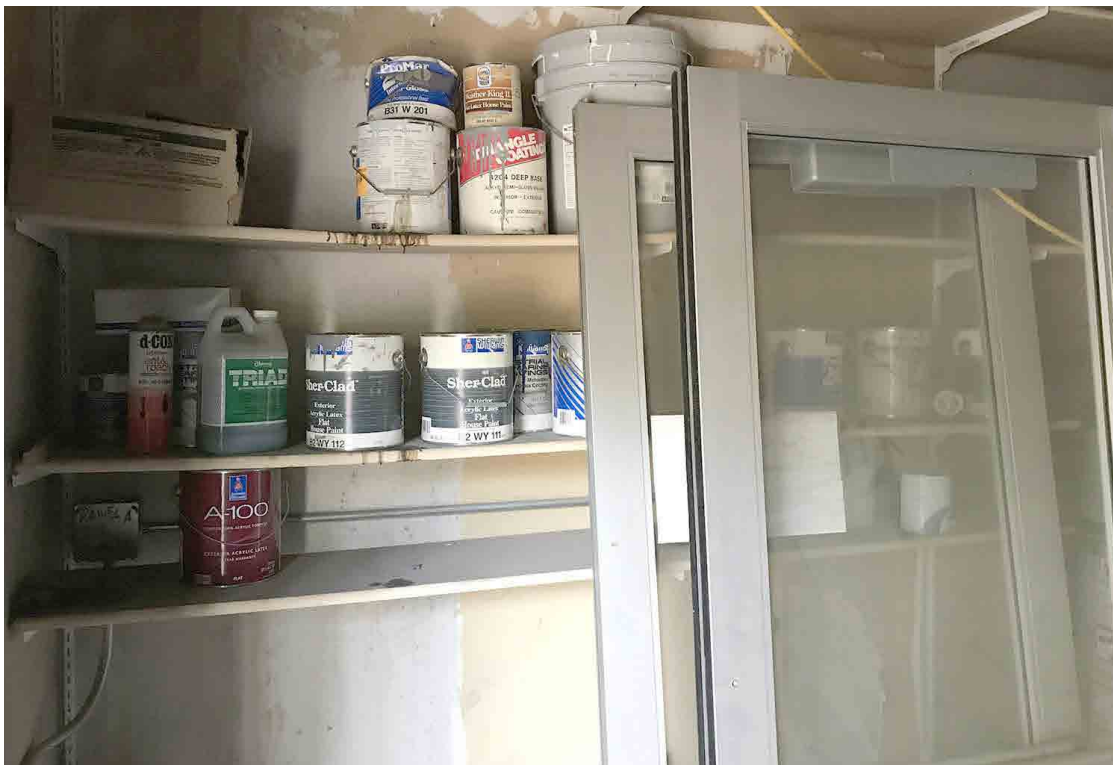
Photo No. 6 Paint storage in electrical room
