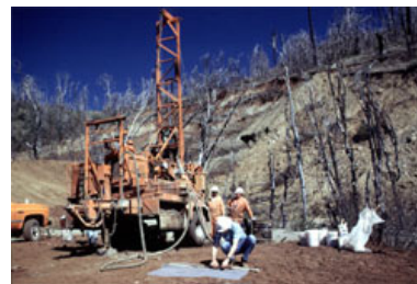
Photo 6: Caltrans drill rig installing subsurface extensometers (to measure landslide movement) and pore-water pressure sensors (to measure ground-water conditions) in the Mill Creek landslide. USGS Photo by Mark Reid, USGS/Menlo Park
