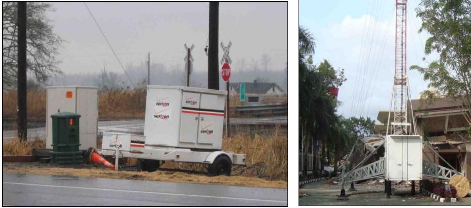
Figure 38. Switch on wheels (left) and cellular on wheels (right) (Photograph taken by A. Tang, L & T Consulting).
