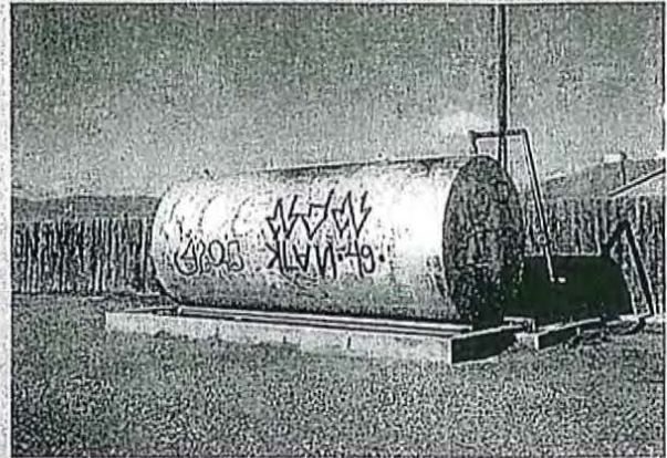
Wrong: This AST has inadequate secondary containment, and no way to prevent vehicles from hitting it.
