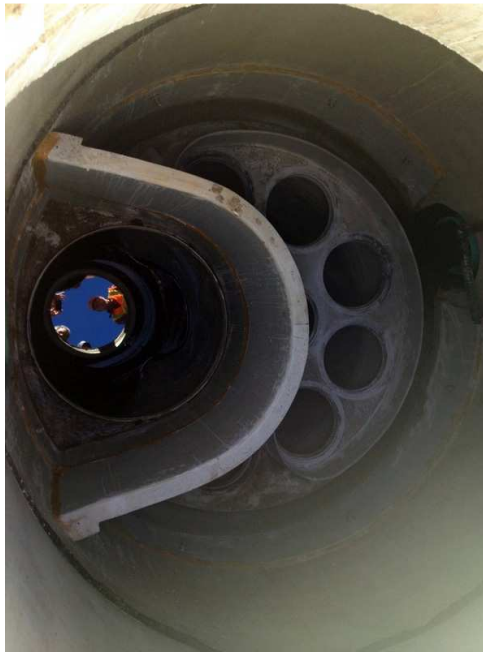
Figure 3: View looking down on Imbrium Jellyfish membrane filtration cartridges installed in concrete vault at SR431.
