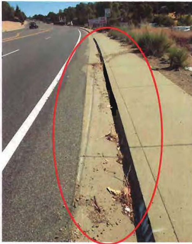
Skid marks and debris from recent accident of vehicle into project site.
