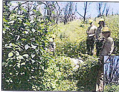
Above: Generation Green crew members prepare to remove dense vegetation from around bedrock milling feature.
