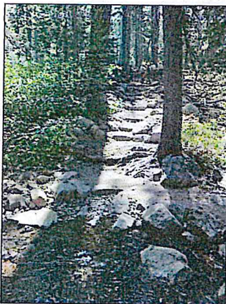
After: Rock steps reduce steepness of grade for reduced erosion and improved user experience, retaining walls on either side of the trail also reduce erosion and stabilize hillsides.
