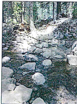
After: large stones for crossing, check steps in trail and platforms to reduce erosion, rock retaining wall and delineation wall between trail and creek to stabilize bank.
