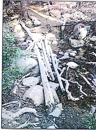
Before: unstable logs for crossing, eroded trail leading to creek, eroded bank between trail and creek.
