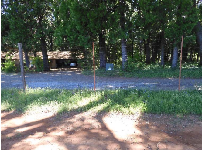
14. View of the power route and the rear transformer from the access road.
