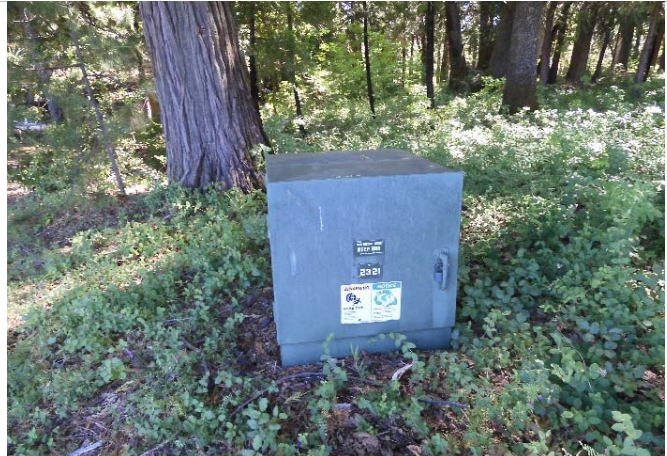
15. View of the power route and the rear transformer from the access road.
