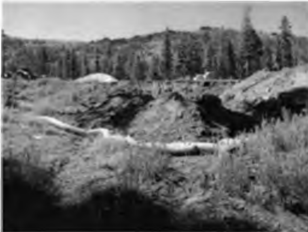
Photo 2. Examples of erosion control material in place during construction of Timber Creek Phase 1.
