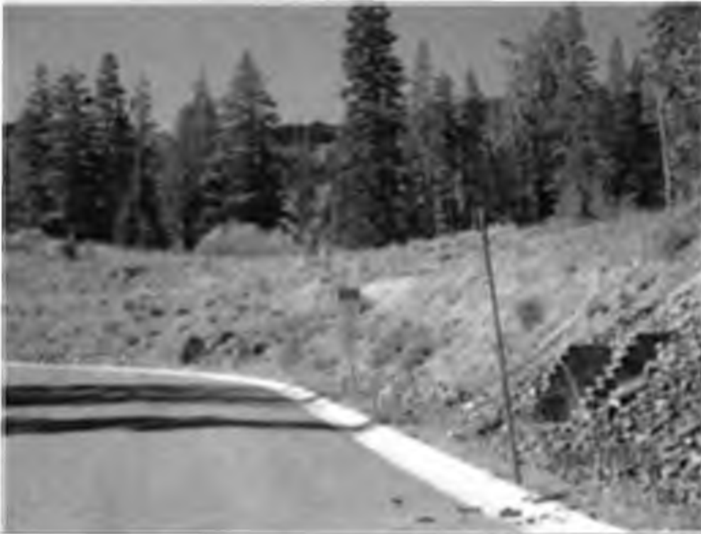
Photo 9. Temporary slope stabilization within Palisades 5. Success of temporary revegetation is variable, but over slope stability maintained by erosion control fabrics and rock as evidenced by lack of dirt and debris on road.
