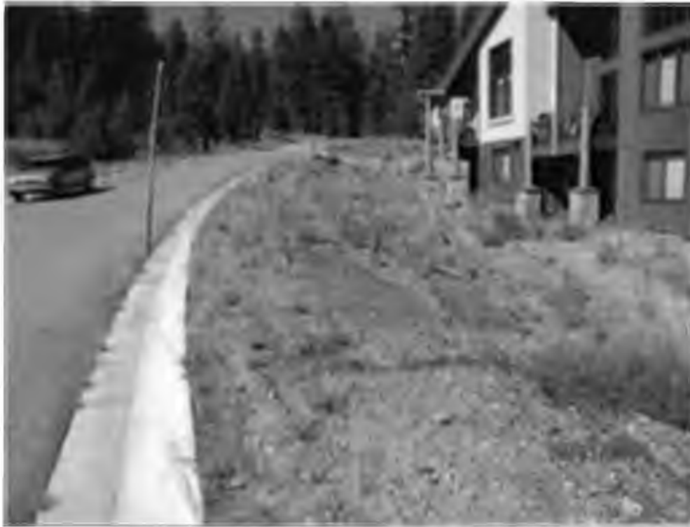
Photo 11. View of failed revegetation along Sentinels Way.
