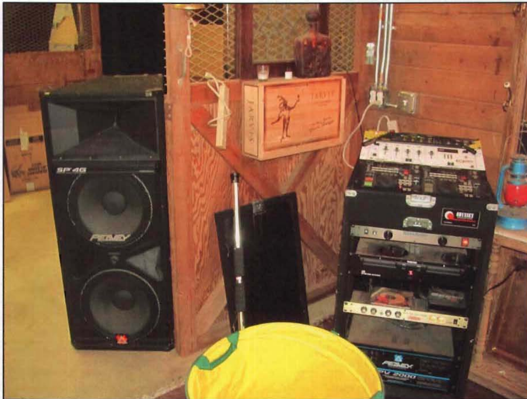
Figure 2 – Sound System within Reception Building
