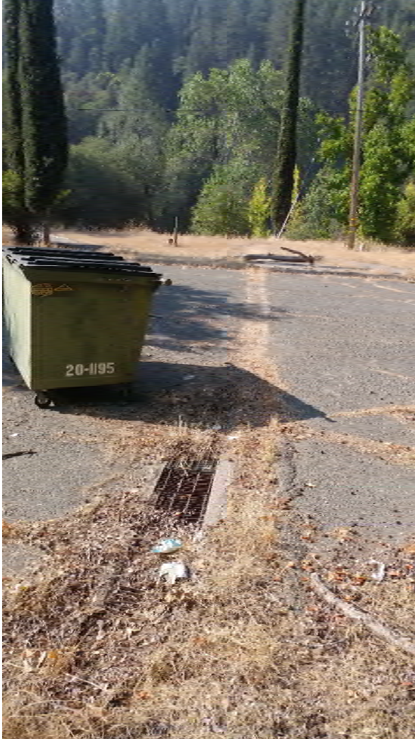
Photo 7 - Trench Drain Filled with Sediment
