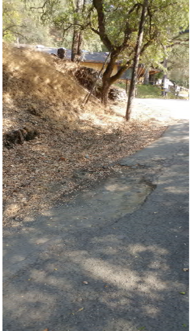
Photo 8 - Road Surface and Drainage Issues
