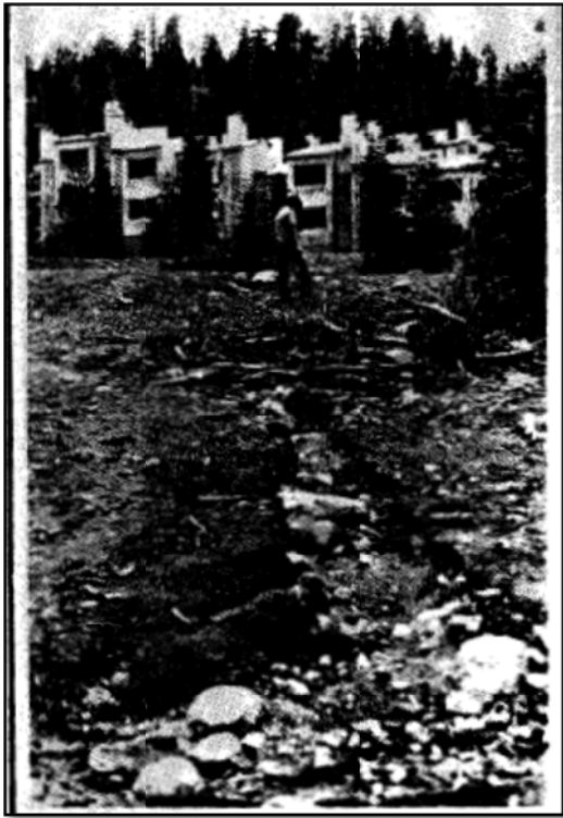
Figure A. Erosion caused by uncontrolled drainage flowing across highly erodible fill area.
