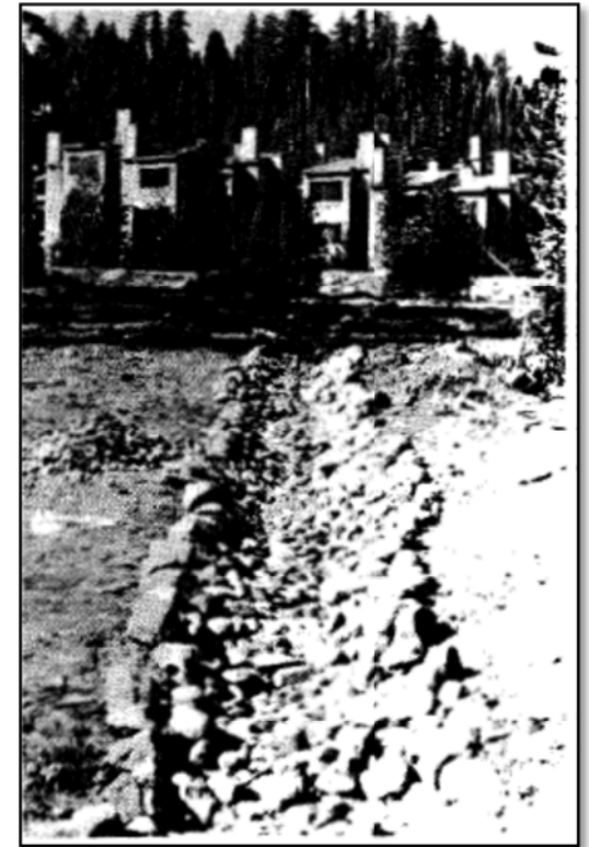
Figure B. Rock lined drainage channel designed to correct problem pictured in Figure A.
