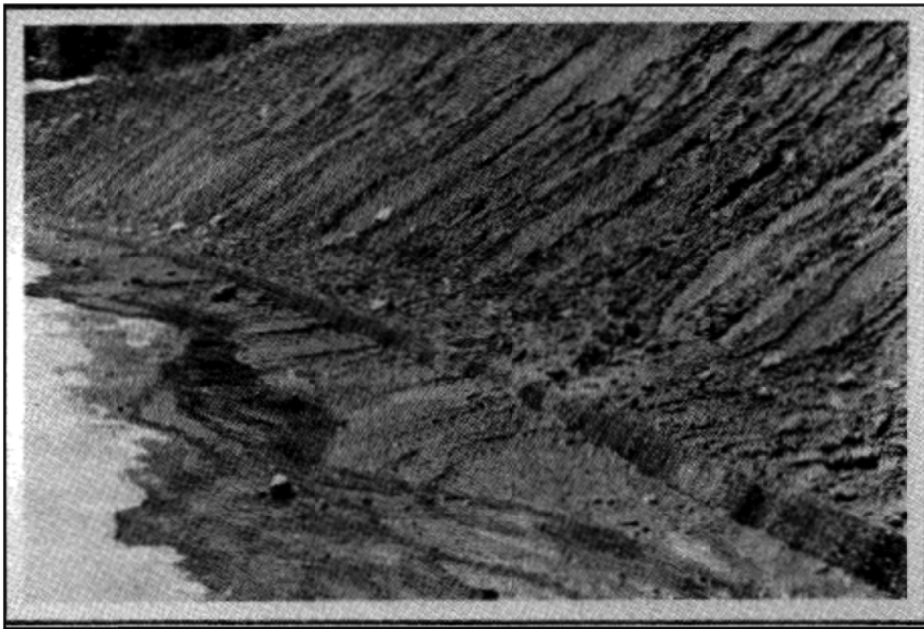
Eroded and accumulated sediments at toe of oversteepened cut slope within Rubicon Properties subdivision. Lake Tahoe Basin, during the summer of 1977.
