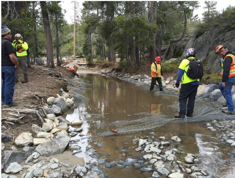
Fencing spread by FOTR volunteers. Rock was dropped on top of the fencing.
