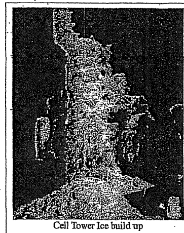
Cell Tower Ice build up
