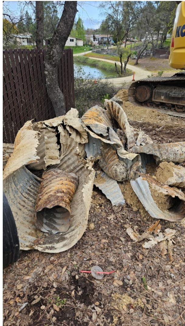
Damaged/destroyed culvert removed from roadway
