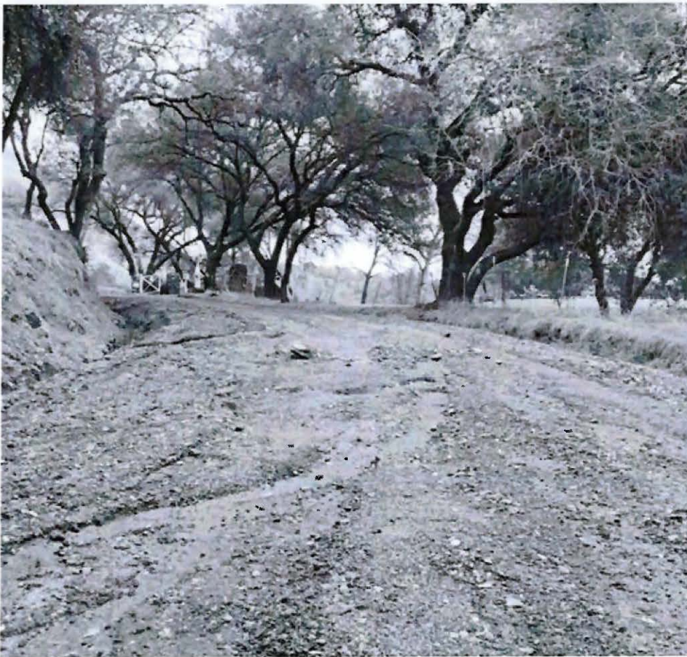
DOT dirt/gravel maintenance atop former HARD SURFACE of road
