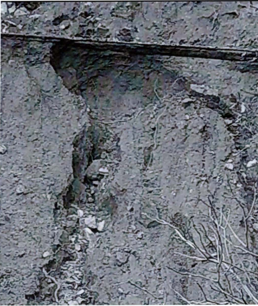
Chunks of SOLID ASPHALT in Mt. Murphy Road strewn length of ditch. Also note loose DOT gravel:
