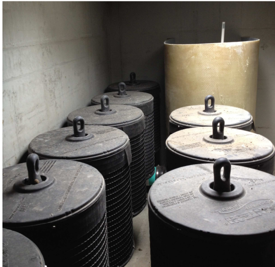
Figure 5: Contech MFS filter cartridges in underground concrete vault at SR431. Float valve is behind fiberglass shield. An outflow pipe runs underneath each row of cartridges.
