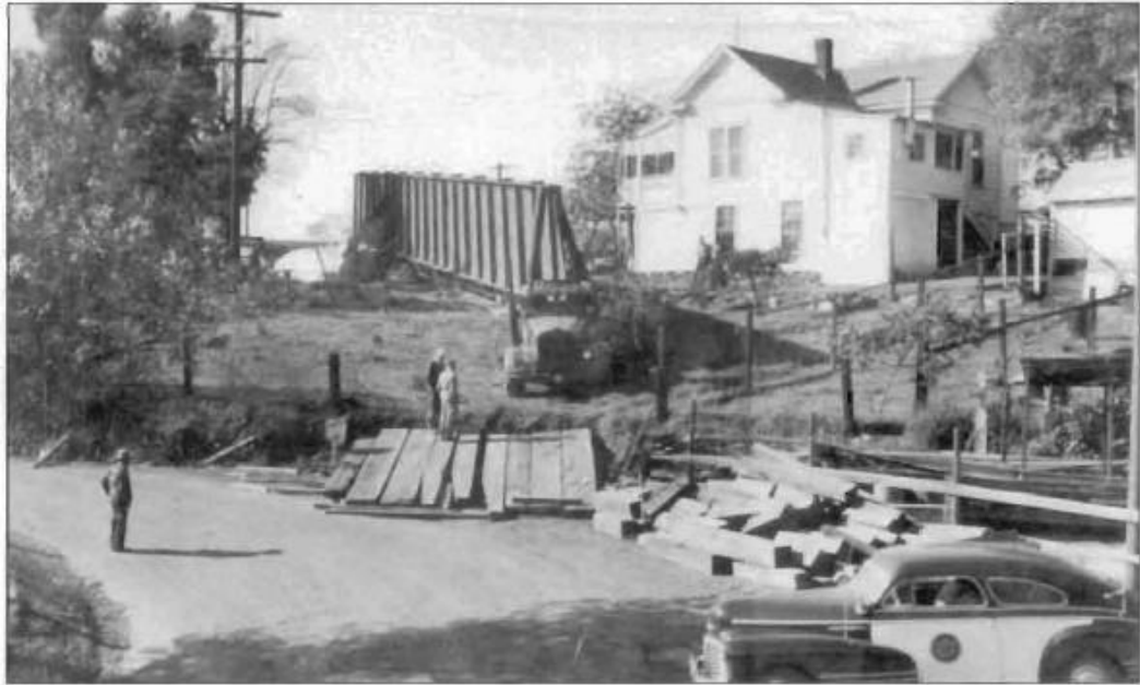
As part of the construction of a new state Highway 49 Bridge on the North Fork, four 60-ton girders were hauled down the canyon. On November 13, 1947, traffic at both ends of the grade was blocked by the California Highway Patrol, while the 127-foot-long girders were transported down the highway. A crane followed along lifting the rear end around tight corners. (Courtesy of the California Department of Transportation.)
