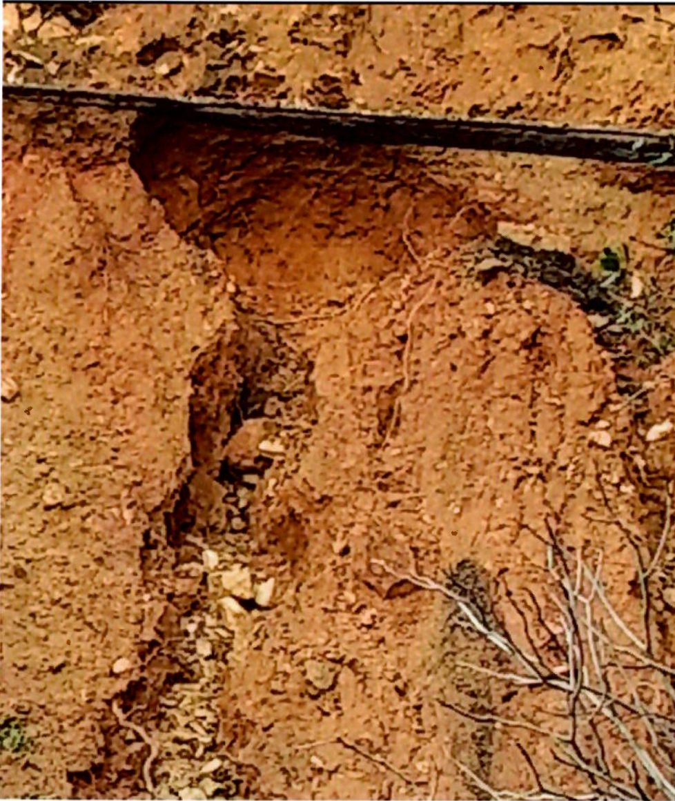
Chunks of SOLID ASPHALT in Mt. Murphy Road strewn length of ditch. Also note loose DOT gravel:
