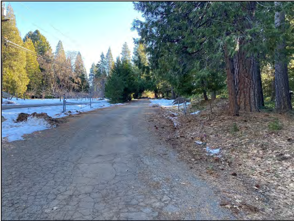
Photo 5. Representative view of Gail Drive in the northern portion of the Study Area within the Developed/Disturbed community. Photo date 1/25/2022.
